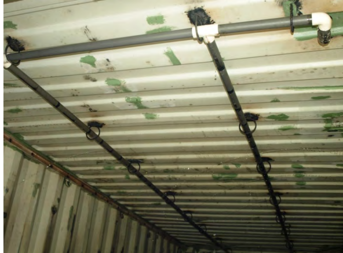
Figure 4: Percolation system inside the container
