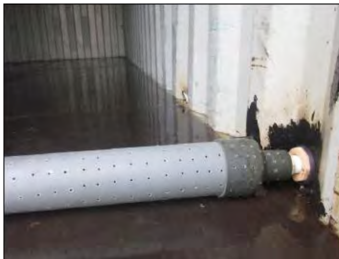
Figure 5: The percolate outlet port (collection pipe)
