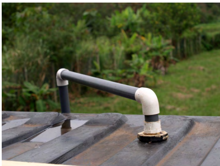
Figure 6: Gas outlet port from the container roof
