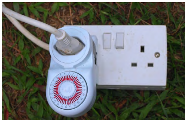
Figure 15: Time switch connected to the pump
