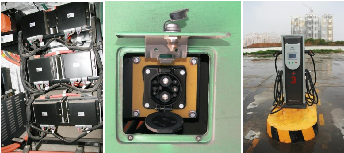
Photos 5: Plug-In Hybrid Electricity Charging (Batteries, Charging Station)
