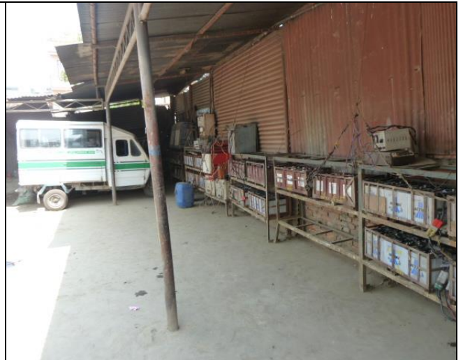
2. Charging station of Umesh Shrestha
