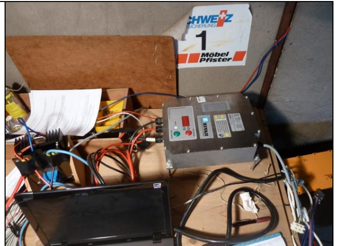
8. Testing of ZIVAN charger
