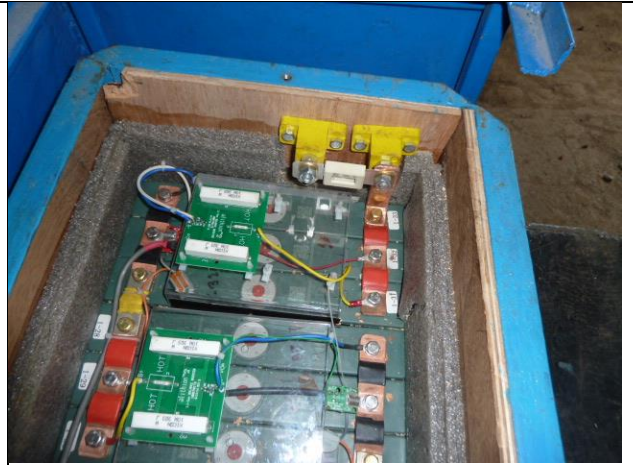
29. Battery box fuse
