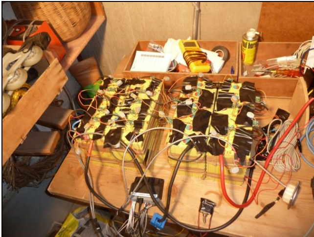
7. Testing batteries, cell boards, BMS controller
