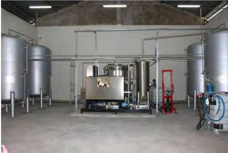
Illustration 5: Fuelmatic GSX 3 biodiesel processor and bulk tank after installation in Bali
