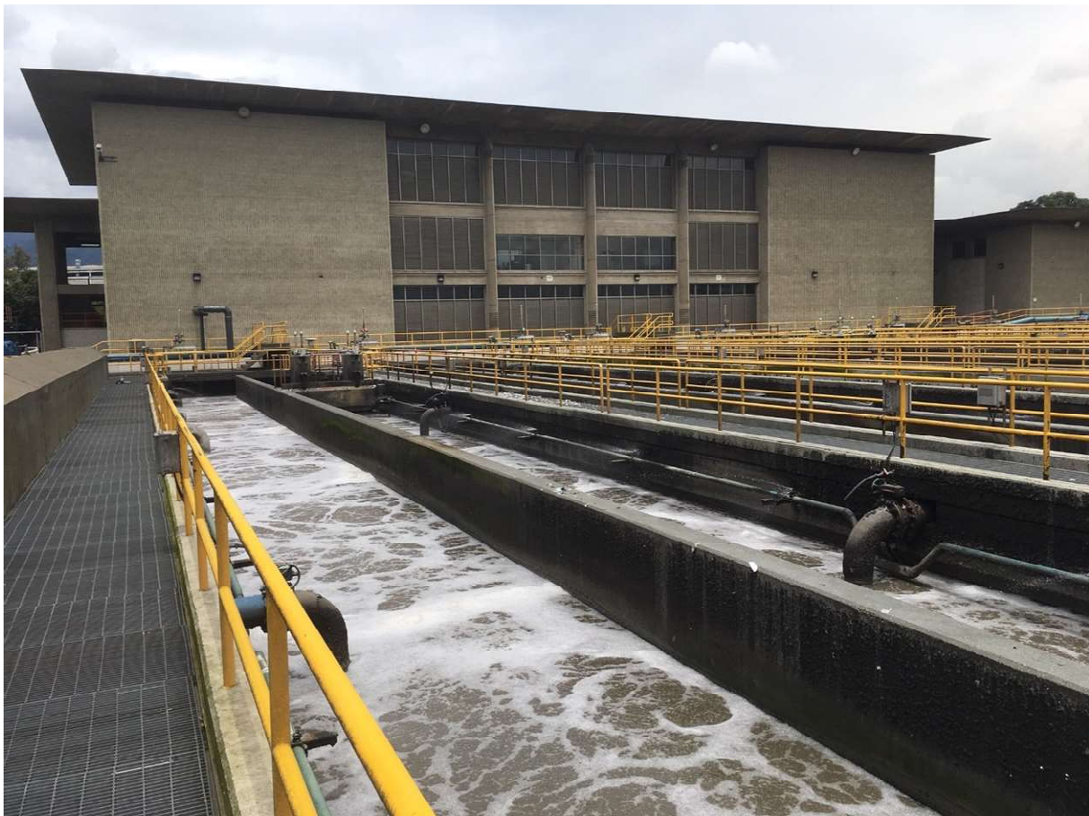
Figure 4 EPM's San Fernando wastewater treatment plant in Medellín with activated sludge basins at the forefront.
