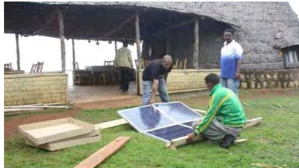
© Sahay Solar Solutions
