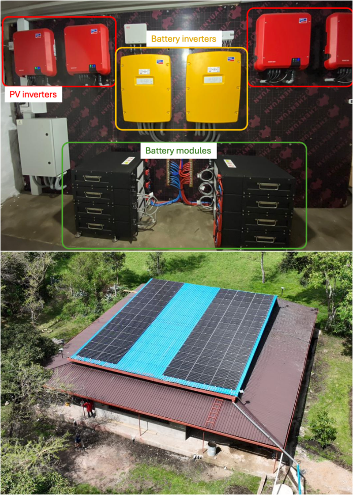
Figure 1: Solar battery system. Top: Inverter and battery installation in underground room. Bottom: Picture of solar PV array on roof of solar mushroom farm.
