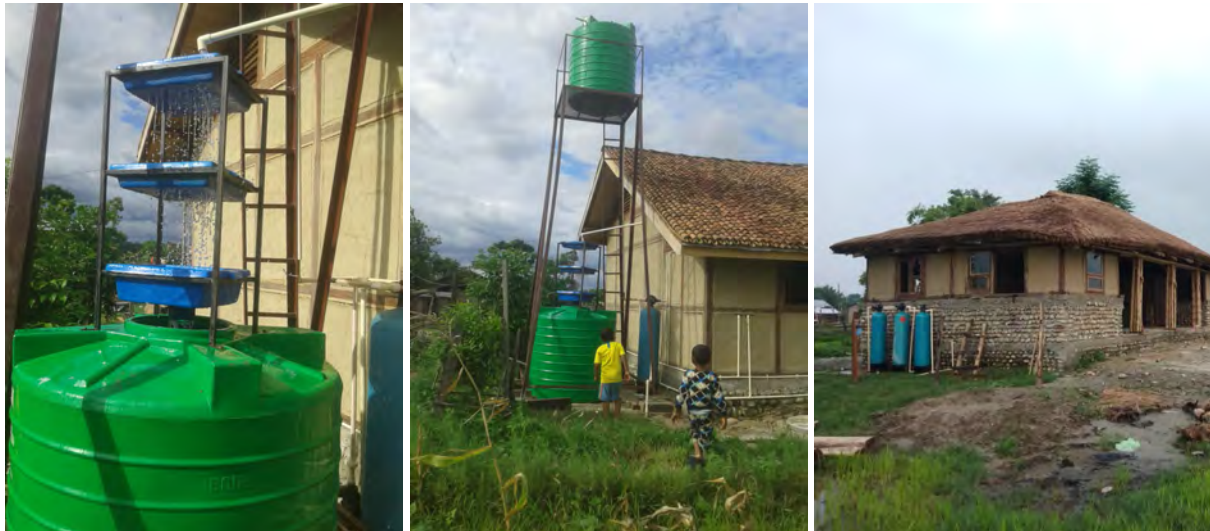
Safe water treatment system: Filtration at homestay (left, mid); Treatment plant at community hall (right)
