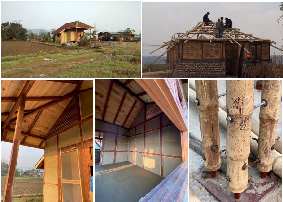
Impressions during construction in March 2021: Homestay (top left) and Community Hall (top right; photo credit: Green Bamboo Creation), with details in wood, mud, elephant grass and bamboo (below).
