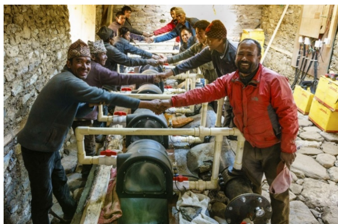
Successful Modular Pico-Hydro Power project partnership between the Mohari village community and RIDS
