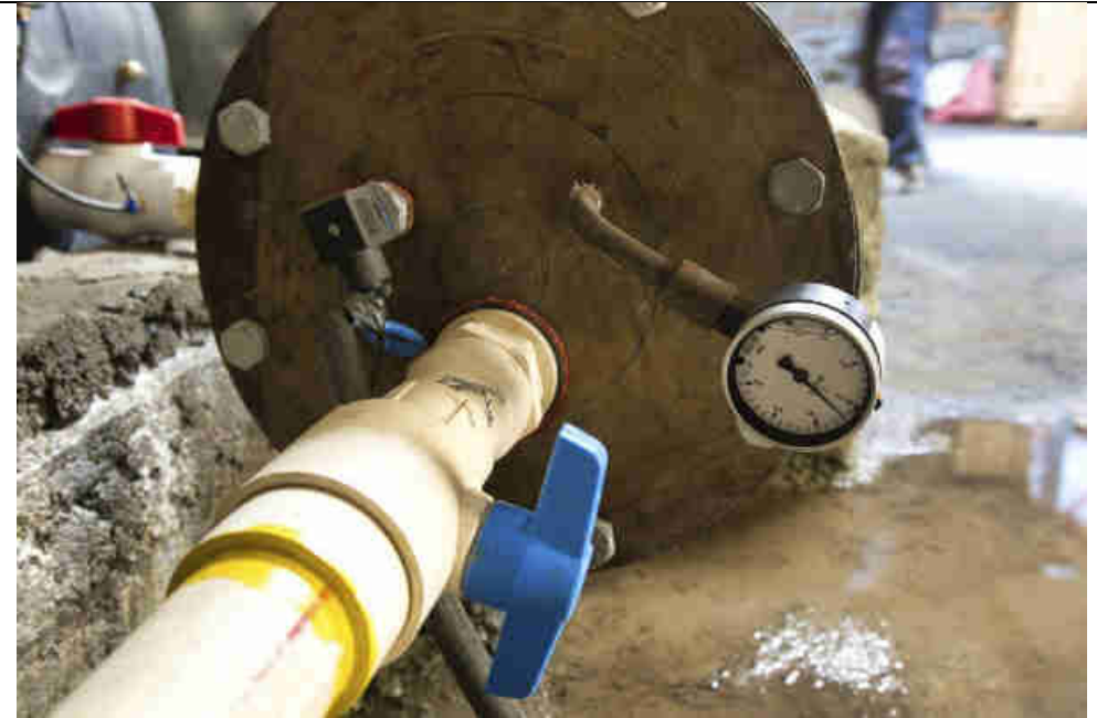
Pic 16: With a Net Head adjusted to 3.4 bar (34m), the 6 turbines generate 4 kW. The blue ball valve is the flush out valve to clean the penstock once a month
