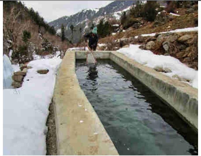
Pic 22: Periodical cleaning of the surface water from leaves and sticks in the sedimentation tank by the operator
