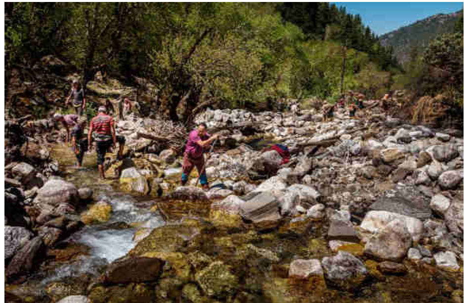
Pic. 78: Diverting the river to be able to build the intake and sedimentation tank
