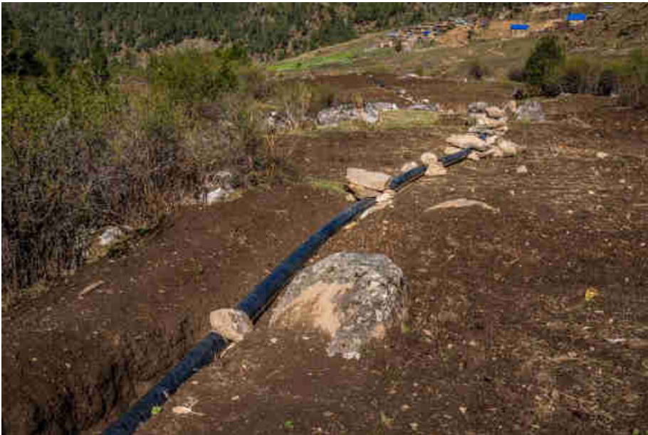
Pic. 57: Joined HDPE penstock ready for the pressure test before being buried
