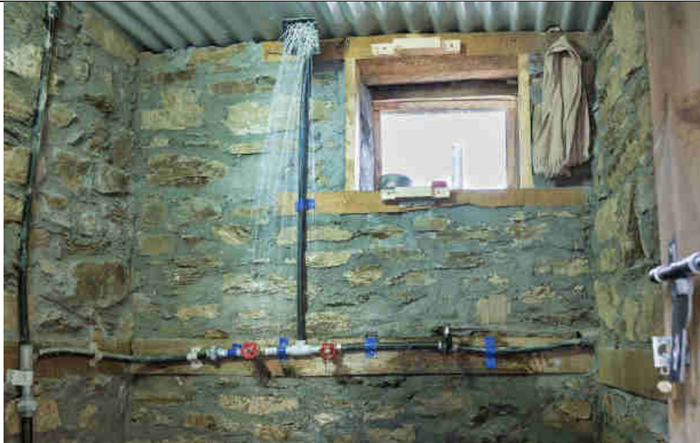
Pic 27: Inside the Power/Community house hot water shower room. The shower temperature can be adjusted from 10 °C (50°F) during no use and winter, up to 55 °C (131 °F) through the Configuration site ( http://www.mohari.rids-usa.org/config.php )
