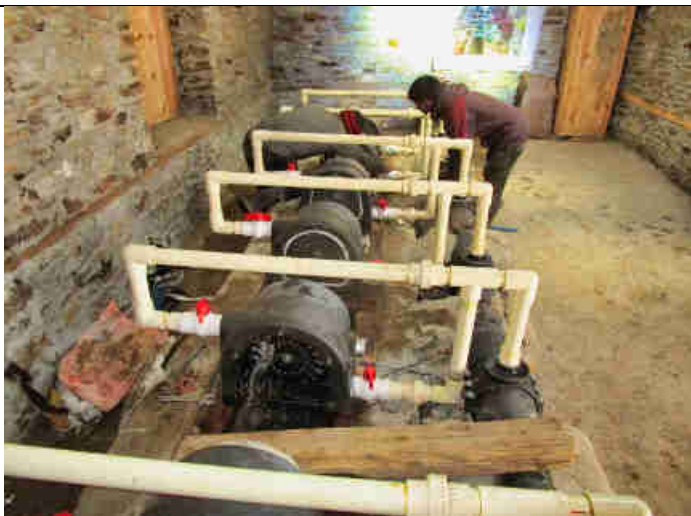
Pic 5: Periodical cleaning and check-up of all 6 Pelton turbines of the Modular Pico-Hydro power plant in Mohari village. This is during the winter even more important than during the other seasons as the way below freezing ambient temperatures cause very harsh conditions for the materials and power plant to run
