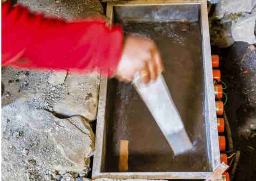
Pic 17: Periodical cleaning of the emergency power dump load in turbine house
