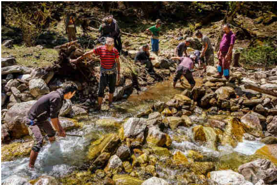
Pic. 77: Diverting the river to be able to build the intake and sedimentation tank
