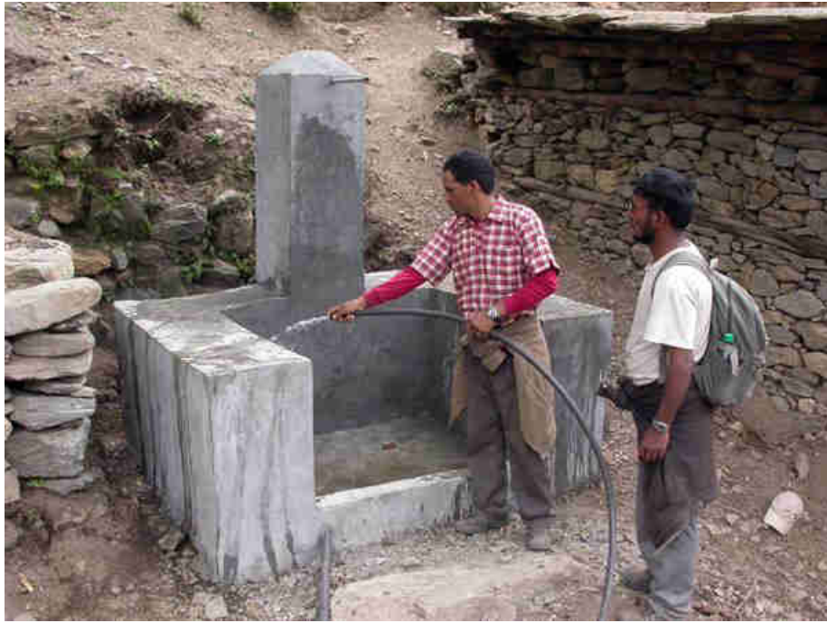
Fig. 9: In close collaboration with RIDS-Nepal the Mohari Village community built its village drinking water system. Water is tapped from their own water source above the village and piped in underground buried HDPE pipes to the various drinking water tap stands distributed in the village according to where they decided they should be.
