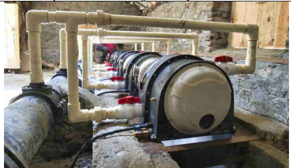
Pic 14: Periodical inspection and cleaning of each turbine, valve and piping system
