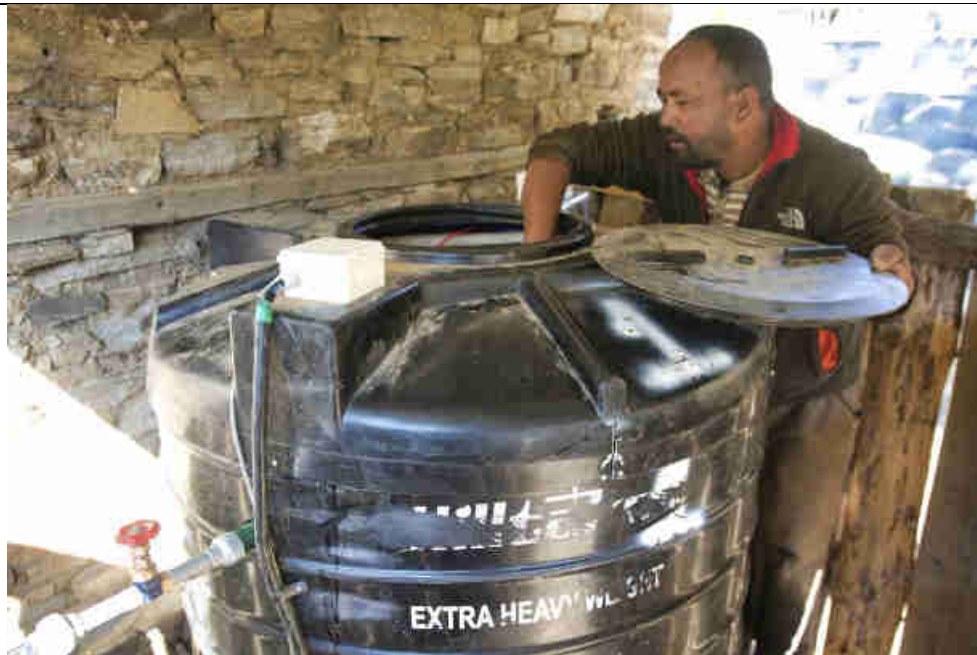
Pic 39: Checking the hot water tank of the village warm/hot shower center
