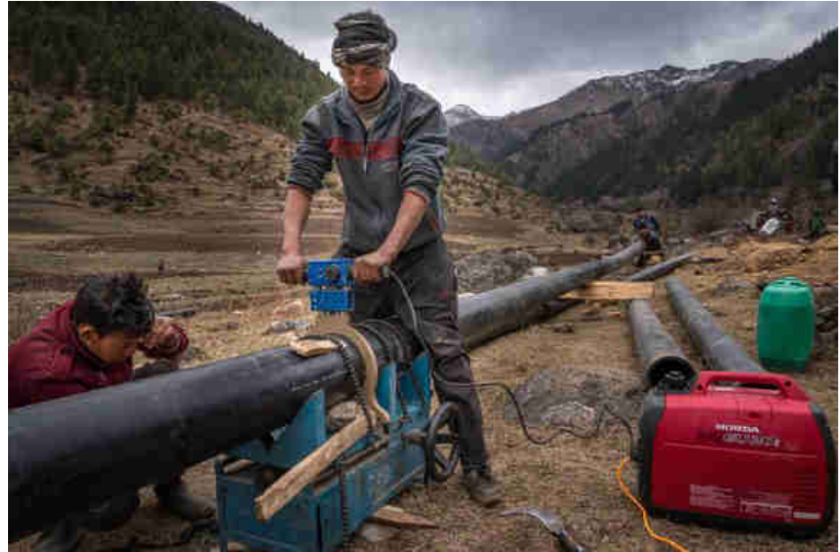
Pic. 40: The HDPE pipes are held in place with chains to assure straightness
