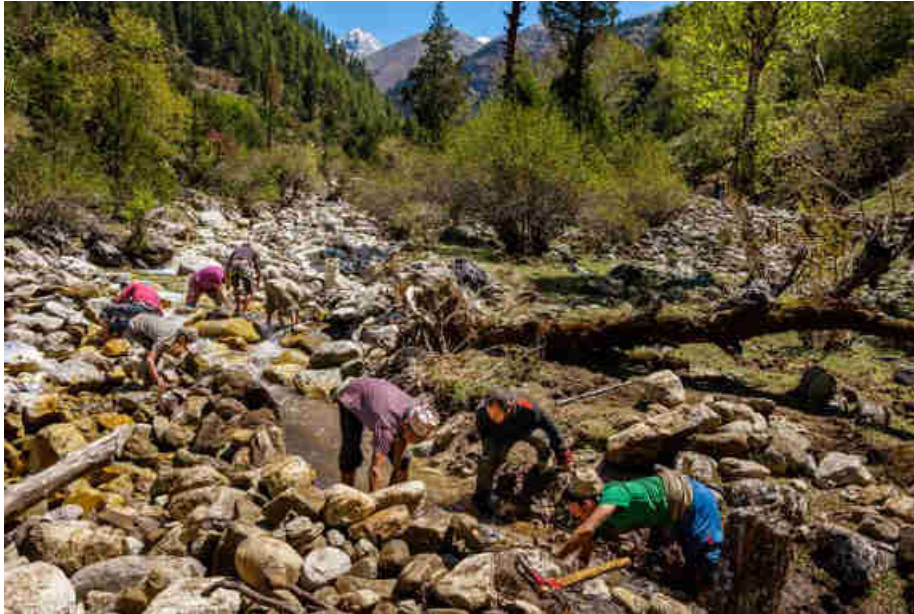
Pic. 79: Diverting the river to be able to build the intake and sedimentation tank
