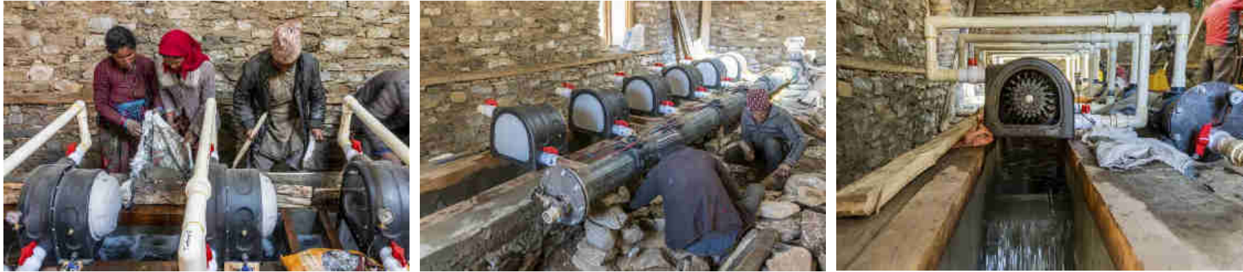
Pics. 64-66: Cementing the water canal for the 6 PowerSpout Pelton Turbines and layout of the penstock and turbines.
