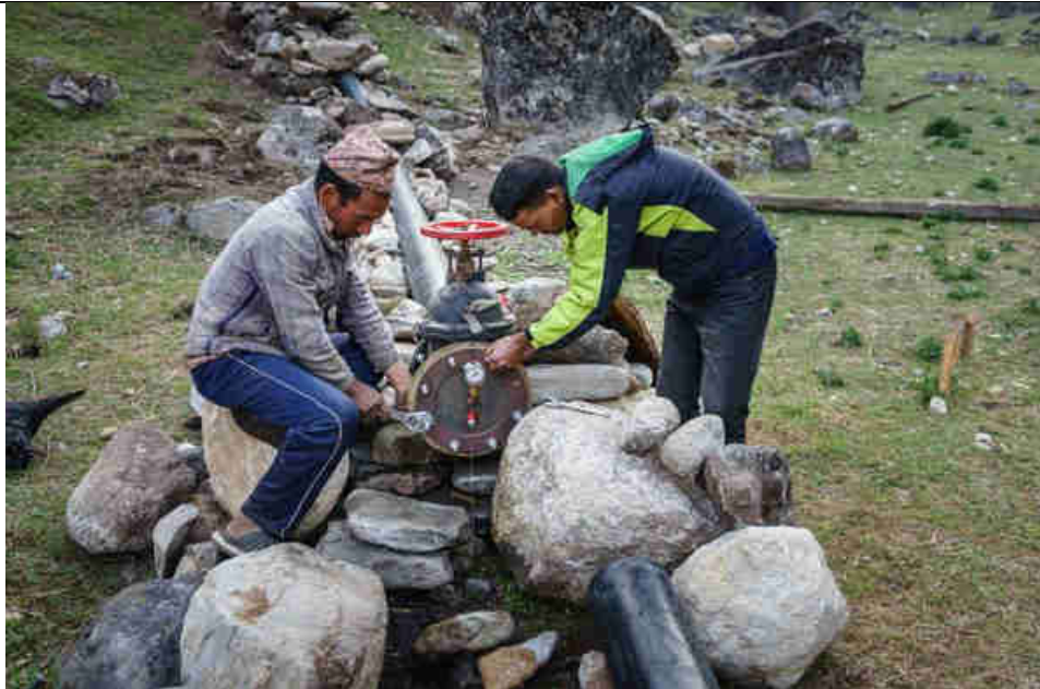
Pic. 12: Successful pressure test of each of the 90 joint-welded HDPE penstock pipes
