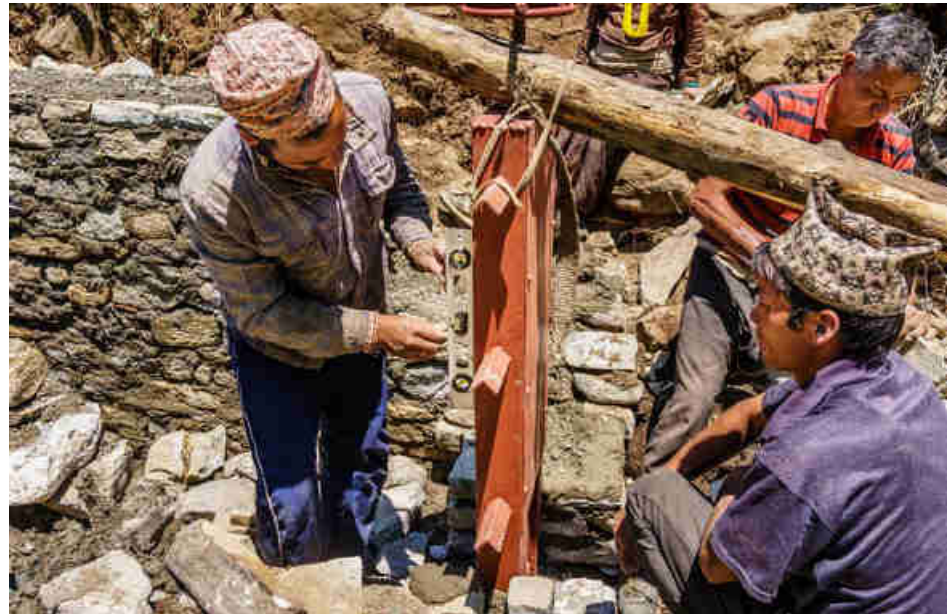
Pic. 90: Installing the sluice gate into the sedimentation tank in correct angles
