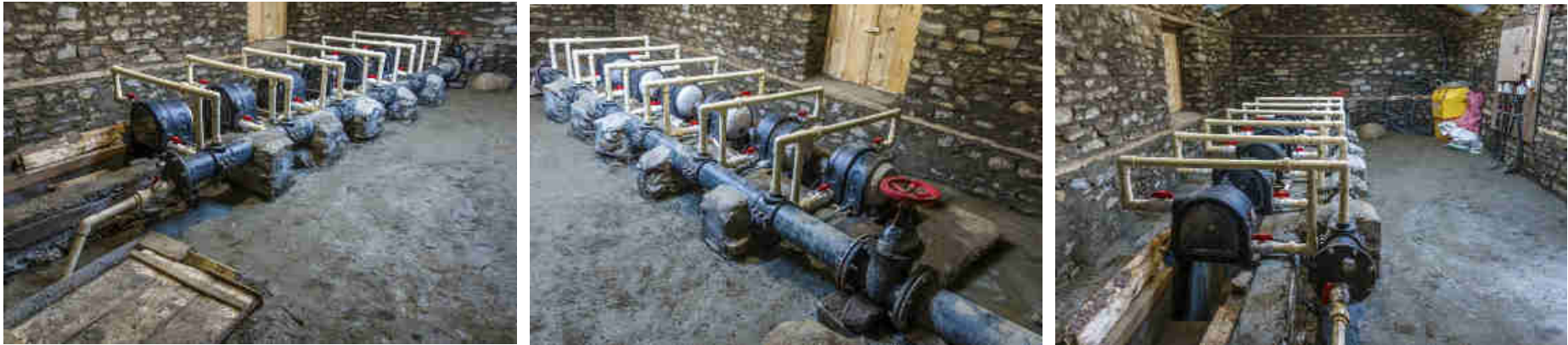
Pics. 4-6: The Mohari Village Modular Pico-Hydro Power Plant with 6 x 1kW PowerSpout Pelton Turbines running in series at 50m head and 24 L/s water.
