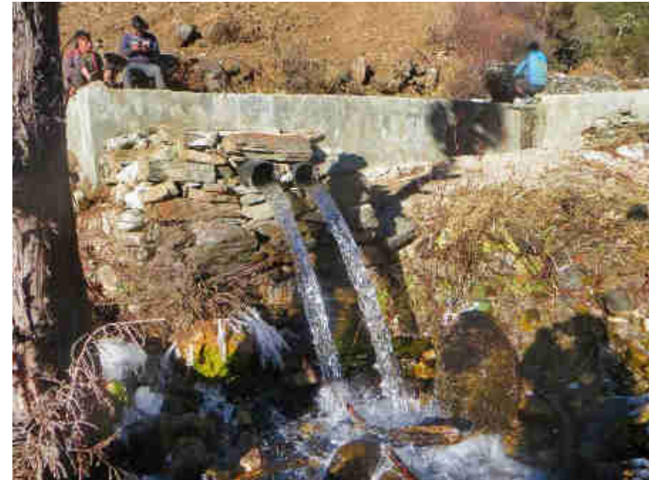
Pic. 6: The sedimentation tank has an overflow, so that the HDP pipe (pic. 5) is always under water and no air can get into the penstock.
