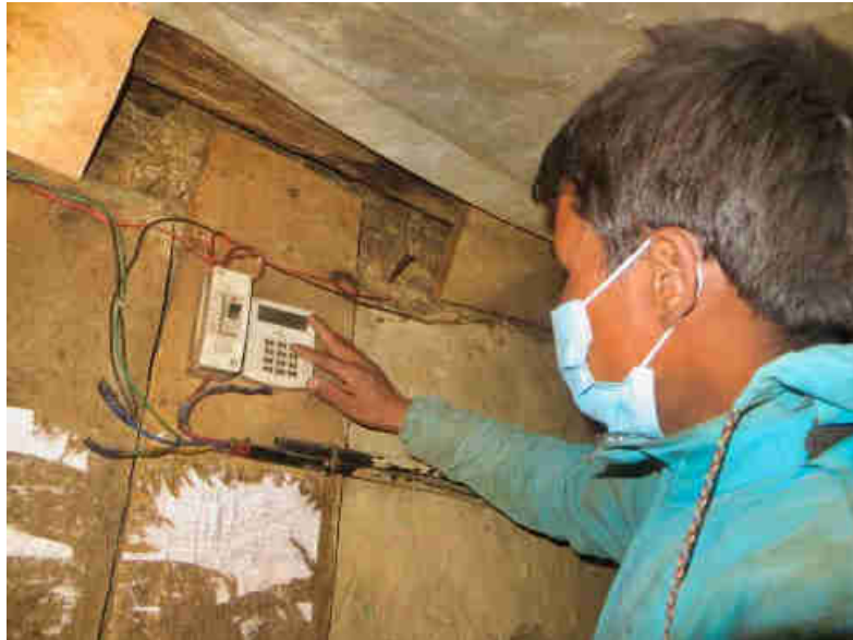
Pic. 23: Hiralal, one of the two trained operators, is recharging a meter box.
