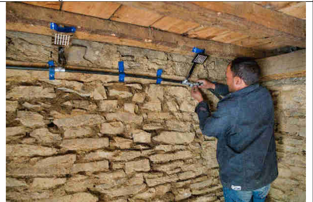
Pic 42: Installation of the shower head in the village based warm/hot shower room
