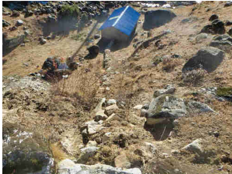
Pic. 7: The underground buried and with boulders covered, 470 m long Ø200mm HDP penstock, leads direct into the Mohari Modular Pico-Hydro Power Turbine house. Gross head is 47m, with a max. water flow of 25 L/sec for all 6 turbines.
