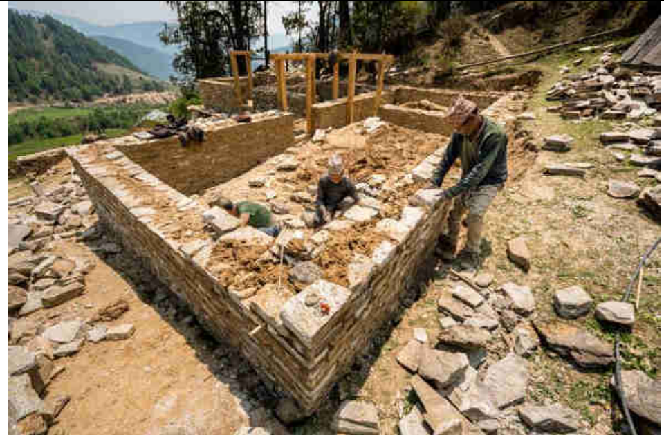
Pic. 17: Building the power house ground walls with stones and mud mortar
