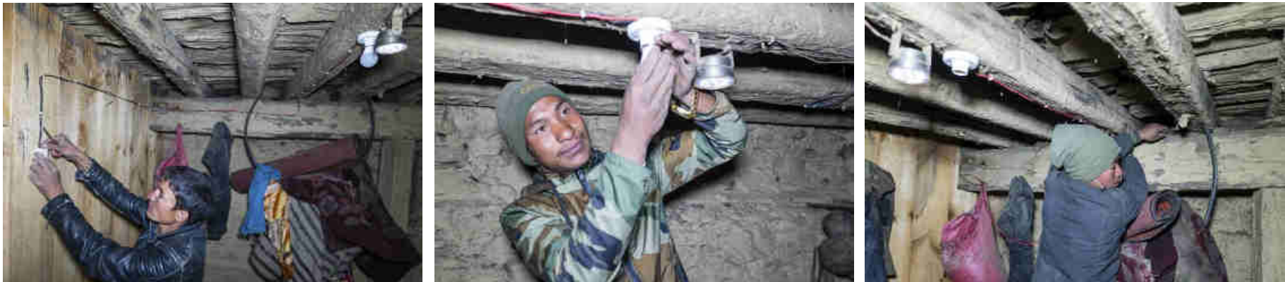
Pics. 37-39: Several local Mohari people have been trained by the RIDS staff in how to install the housewiring system, the cables, the LED lights, MCB (maximum current breaker) and switches.
