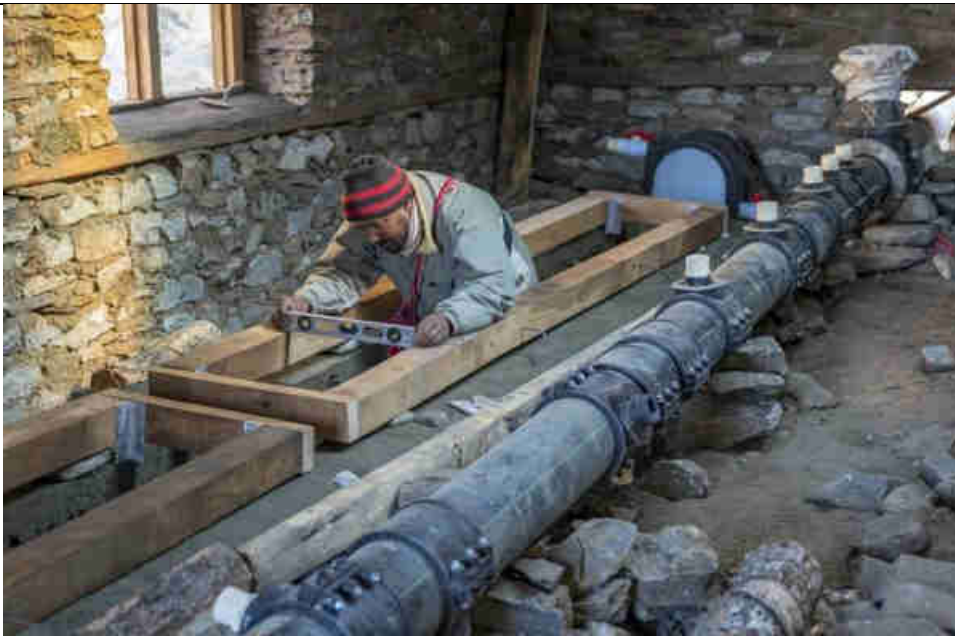
Pic. 20: Building the water canal for the 6 Pelton Turbines inside the turbine house
