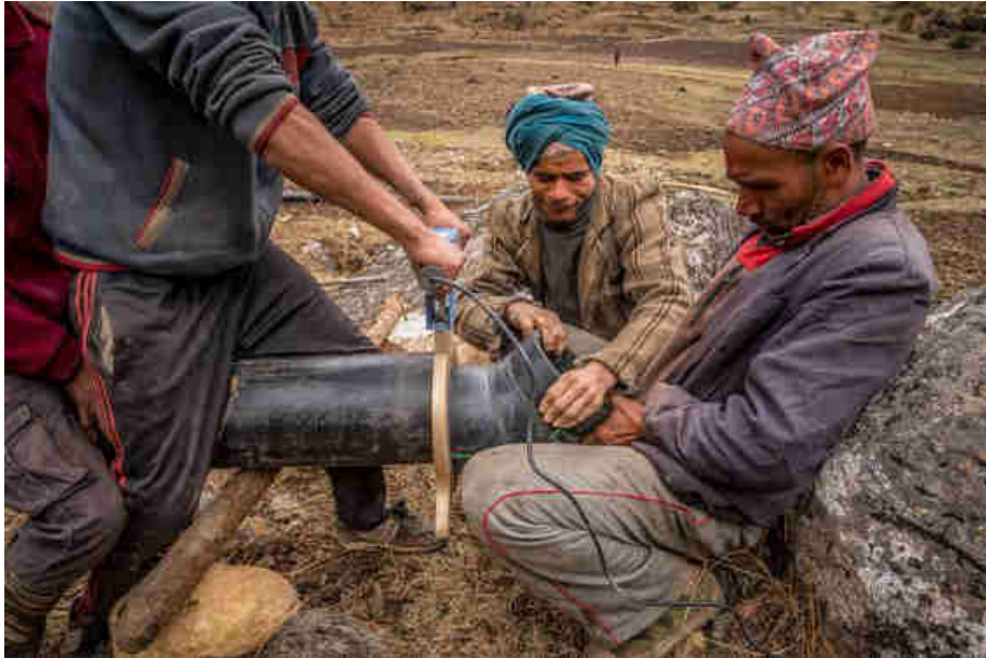
Pic. 47: Welding on a 45° HDPE elbow to assure the correct drop of the pipeline
