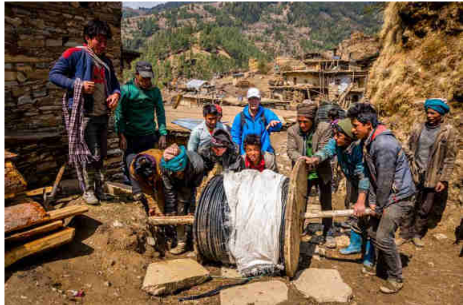
Pic. 26: Unrolling the underground cable from the turbine to the power house
