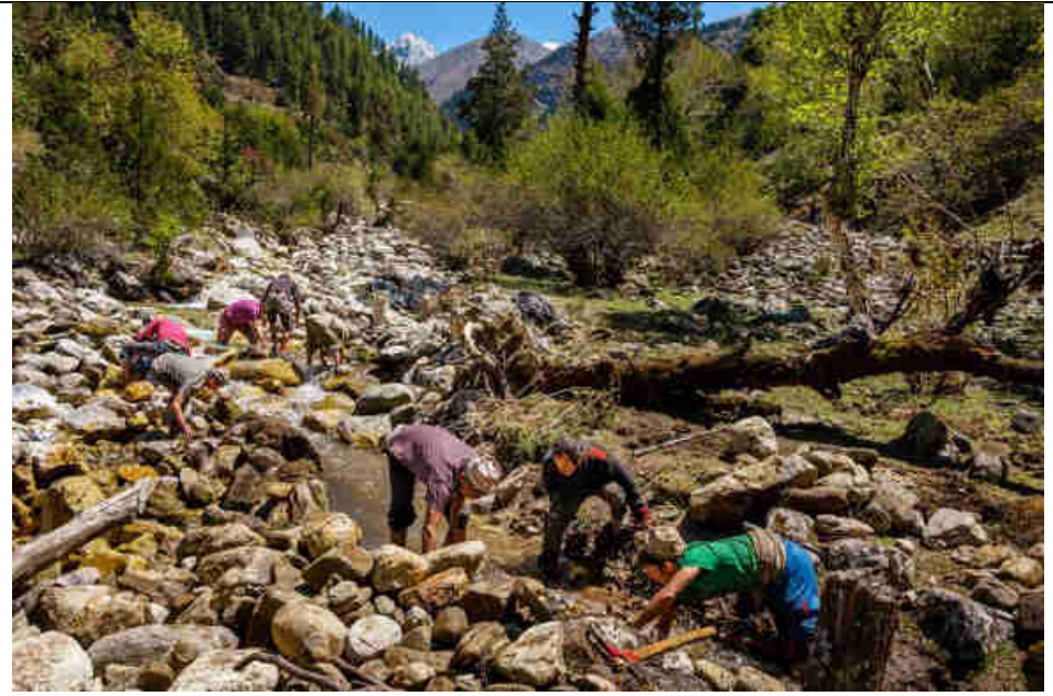
Pic. 13: Diverting the river to be able to build the intake and sedimentation tank
