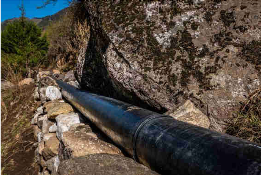
Pic. 55: HDPE penstock on a stone bridge for a gradual, continuous slope
