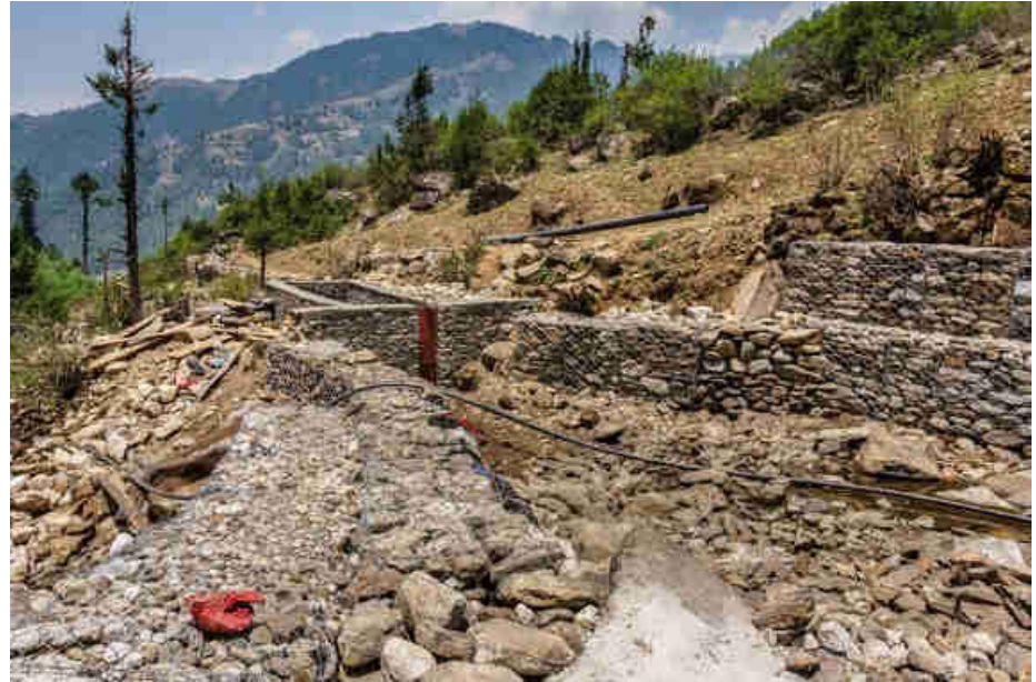
Pic. 92: Gabon wire boxes protection for the sluice gate and sedimentation tank
