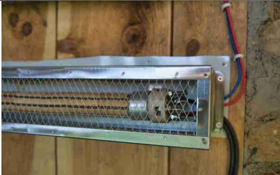
Pic 63: The “smart” dump load room heaters are 48VDC resistive heaters which use power not immediately needed by the village but generated by the modular pico-hydro plant. The pico-hydro power plant’s PC software allocates the various power demands, set based on different user energy service demand priorities, in real time
