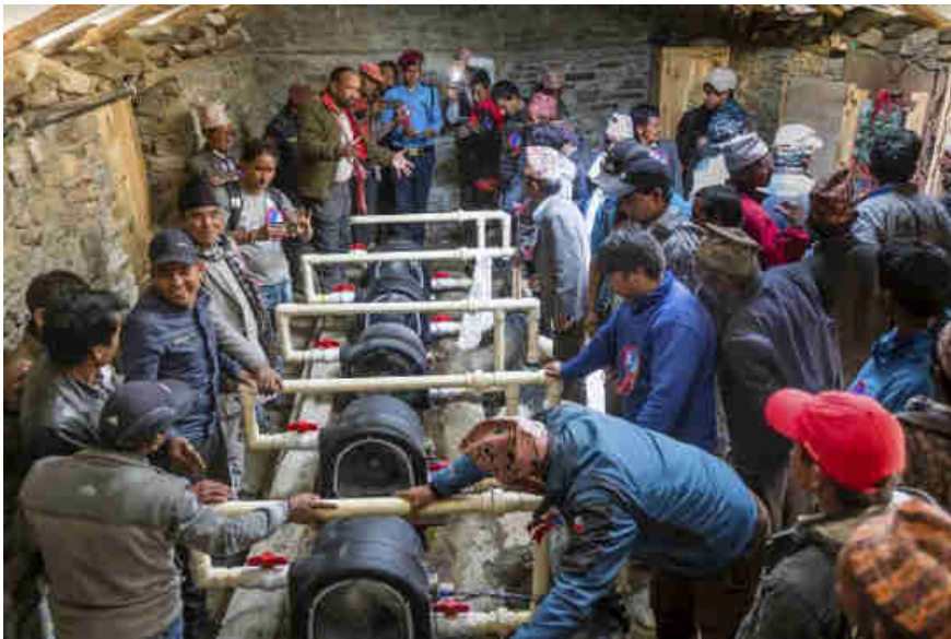
Pic: 42: Inauguration of the Mohari modular pico-hydro power plant on 21 st June 2019
