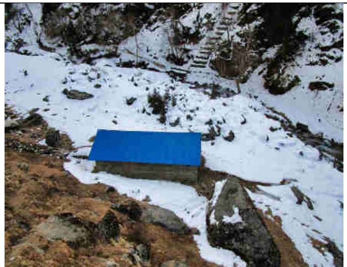
Pic 18: The Modular Pico-Hydro Power Plant Turbine house with the 6 Pelton turbines inside generating 24/7 up to 6.6 kW electricity when all 6 turbines run at their maximum power output (47 meters head and ~3-liter water per second per turbine)
