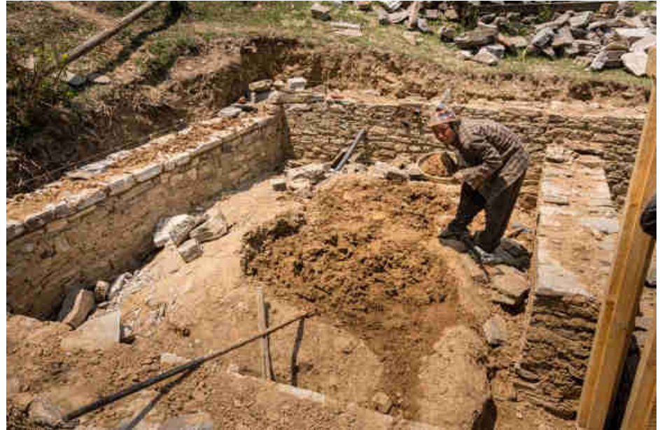
Pic. 120: Mixing mud with water for “mortar” for building the ground walls
