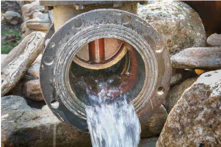
Pic. 69: Successful pressure test (5bar) of te gate valve at the turbine house entry
