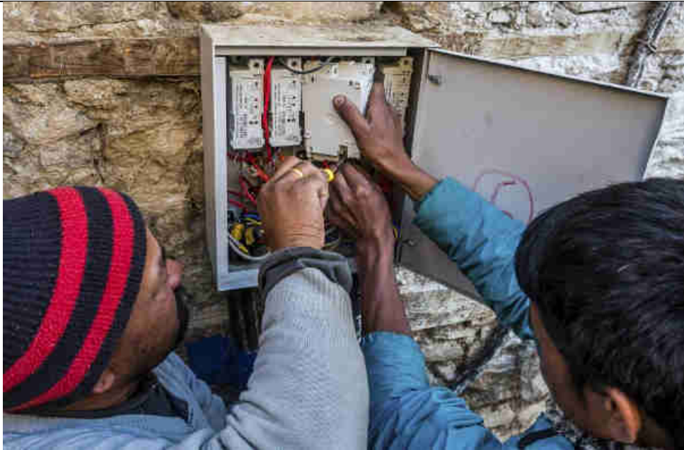
Pic 31: Installation of the smart meters in the various junction boxes in the village
