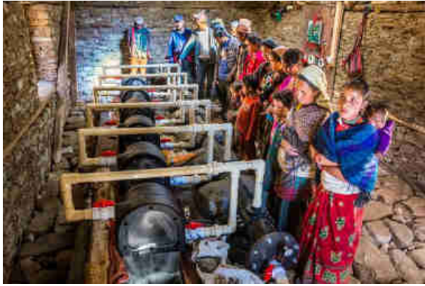
Fig 5: Six Turbines, Saddles, and CPVC Supply Lines
