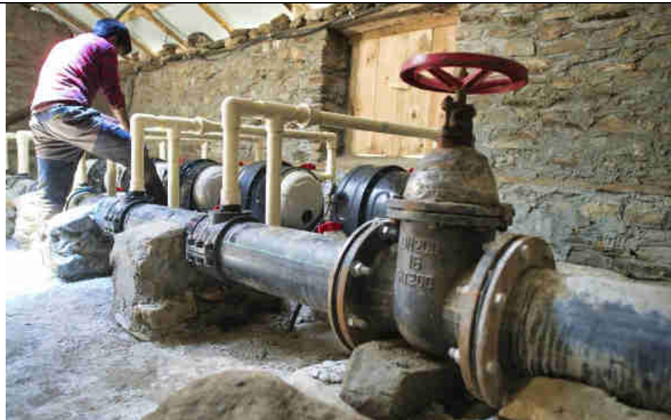
Pic 13: Monthly inspection and maintenance of each turbine and piping system
