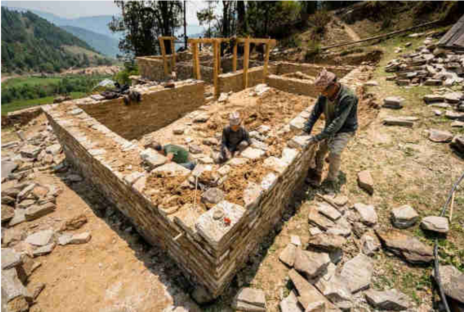
Pic. 111: Building the power house ground walls with stones and mud mortar
