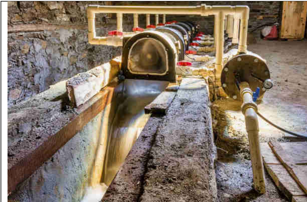
Pic 7: There is place, sufficient water and cable capacity for additional 2 turbines
