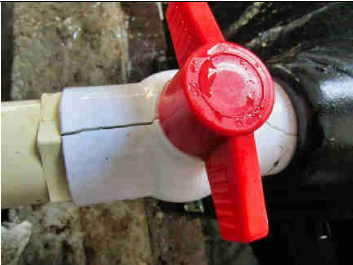
Pic 3: A closed turbine nozzle ball valve caused the water to freeze inside the valve, cracking the hard plastic ball valve body
