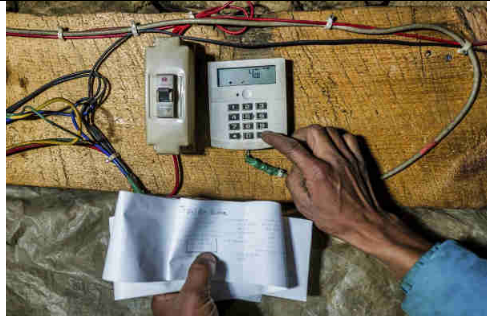
Pic 36: Once the token number issued by the PAYG system is accepted, the display shows the new energy the user has left.
