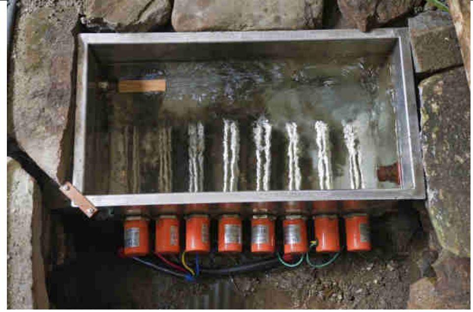
Pic 18: Cleaned emergency power dump load (up to 8 kW) in turbine house
