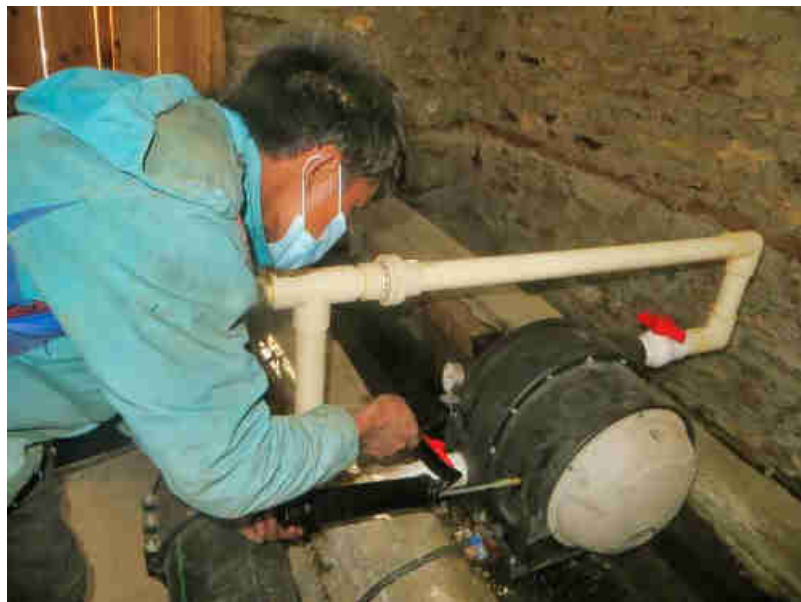
Pic. 9: Hiralal during the monthly periodical maintenance of the pico-hydro power plant. Here he is greasing of each of the 6 Pelton turbines' generator axes.
