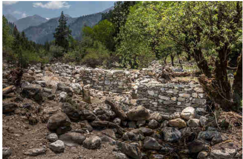
Pic. 86: Ensuring that the river in the rainy season is not endangering the intake
