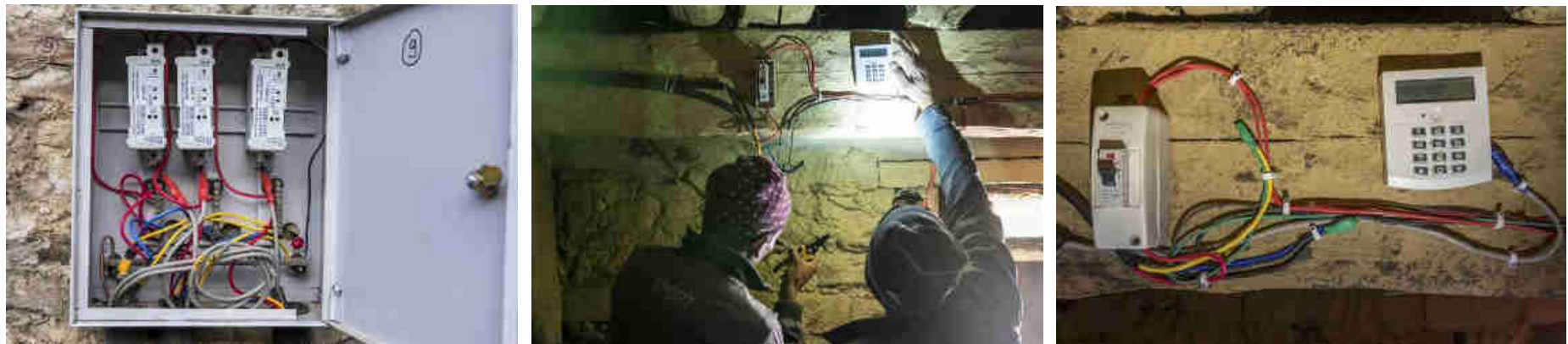
Pics. 49-51: Installation of the 11 different distribution boxes in the village (left) with the PAYG meters for each household. Installation of each MCB and pre-payment display box in each home (middle and right).
