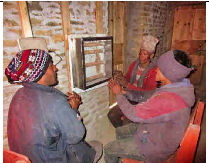
Pic 24: Warming up in front of the "smart dump room heaters" in one of the rooms in the Mohari village Community/power house before heading back out again for work
