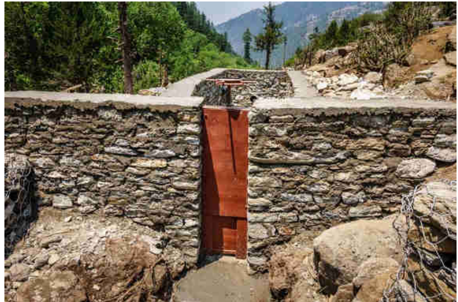
Pic. 94: The sluice gate is the entry gate and protection to the sedimentation tank
