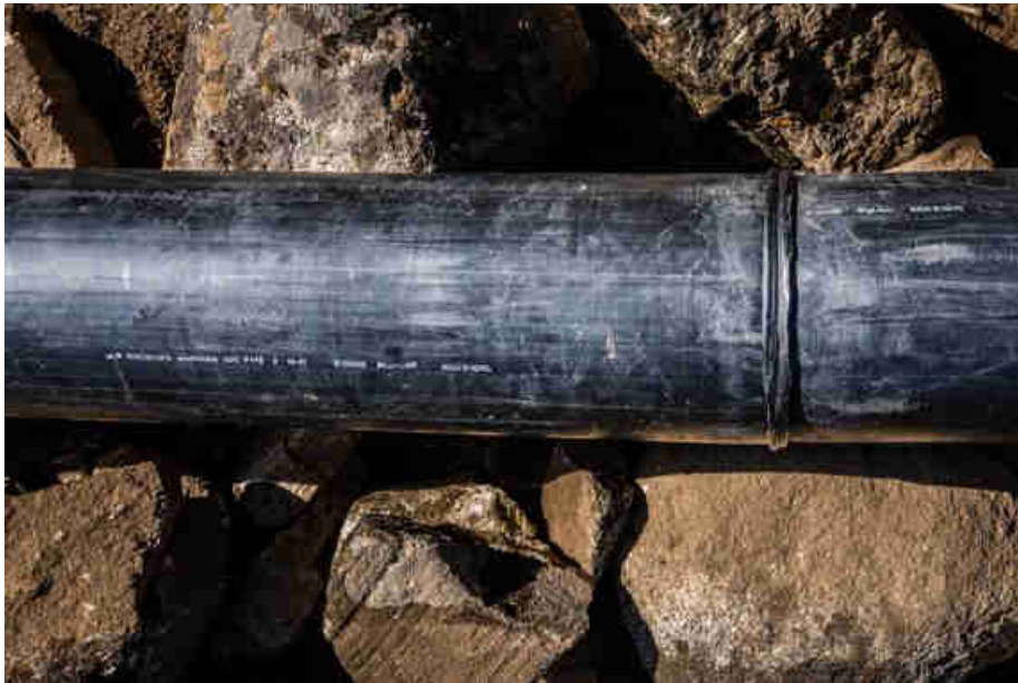
Pic. 45: A close up of one of the 91 joints of the HDPE penstock pipes
