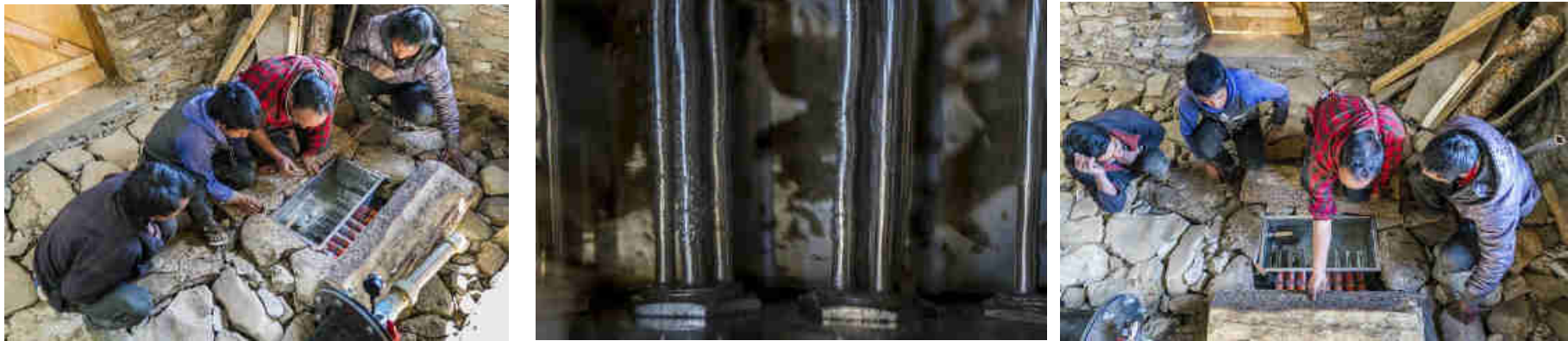
Pics. 76-78: Emergency, 8 kW resistor water heater in the turbine house. This emergency heater is used ONLY if all the other, normal user loads and all the other “smart dump loads” (warm water bathing center, biogas digester heater and room heaters in the power/community house) are NOT in use due to a technical problem in the power transmission line from the turbine house to the power house.
