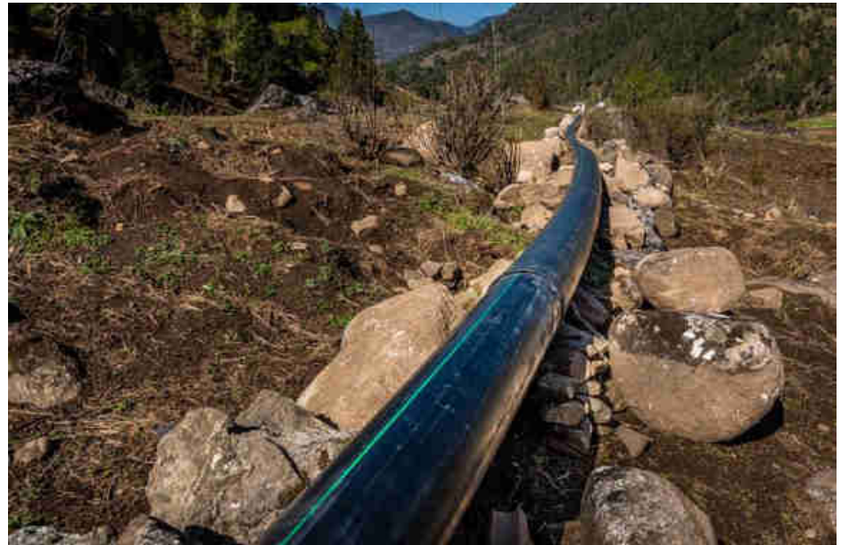
Pic. 58: Welded HDPE penstock ready for the pressure test before being buried
