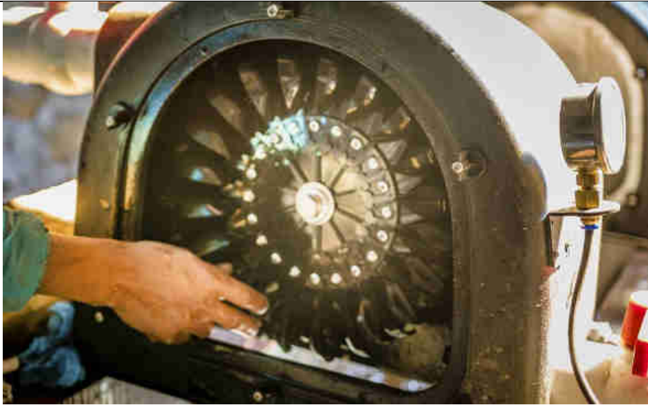
Pic 11: Monthly inspection of the Pelton turbine
