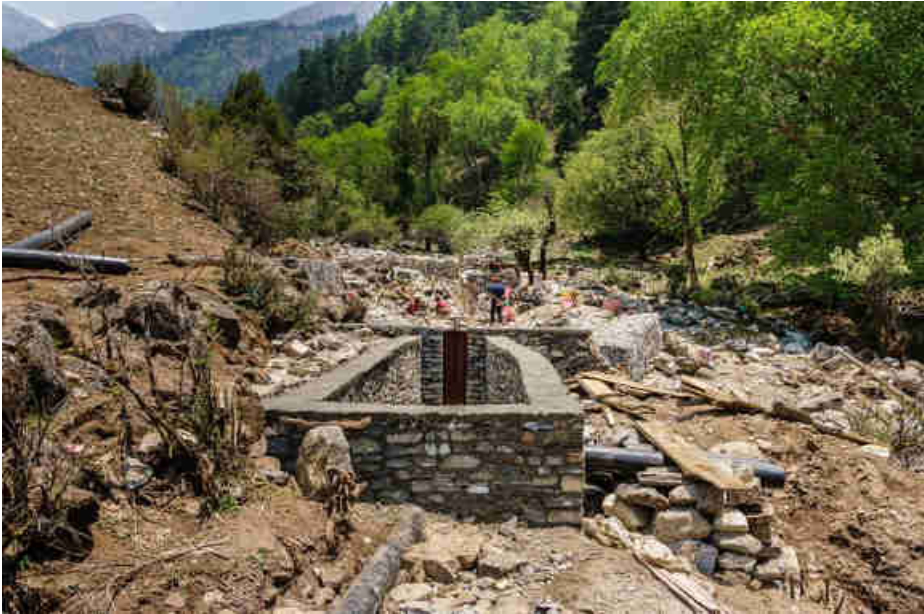
Pic. 95: River, gabon wire protection boxes, sluice gate and sedimentation tank
