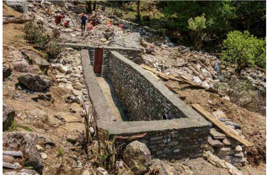
Pic. 96: : River, gabon wire protection boxes, sluice gate and sedimentation tank
