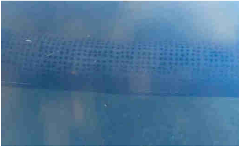
Pic. 5: A Ø200 mm HDP pipe with over 1'600 holes with Ø8mm in the sedimentation tank prevents any small debris to be sucked into the 470 m long penstock. That protects the 6 Pelton turbines in the turbine house (pic. 7 & 10).
