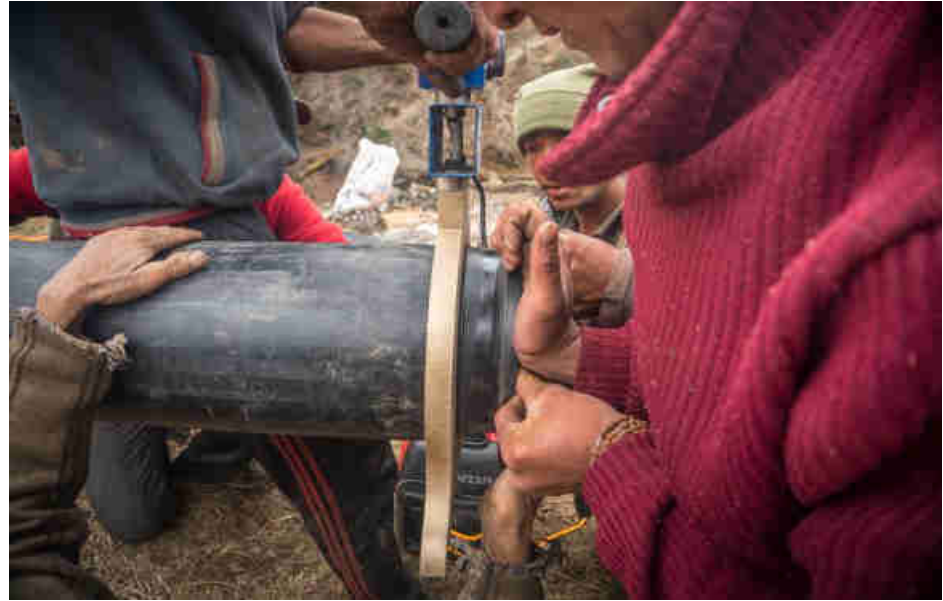
Pic. 48: Welding on an HDPE flange to connect the expansion HDPE pipe
