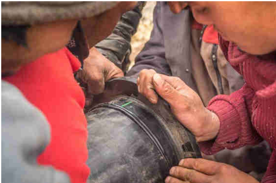
Pic. 49: Welding on the HDPE flange to connect to the flange set
