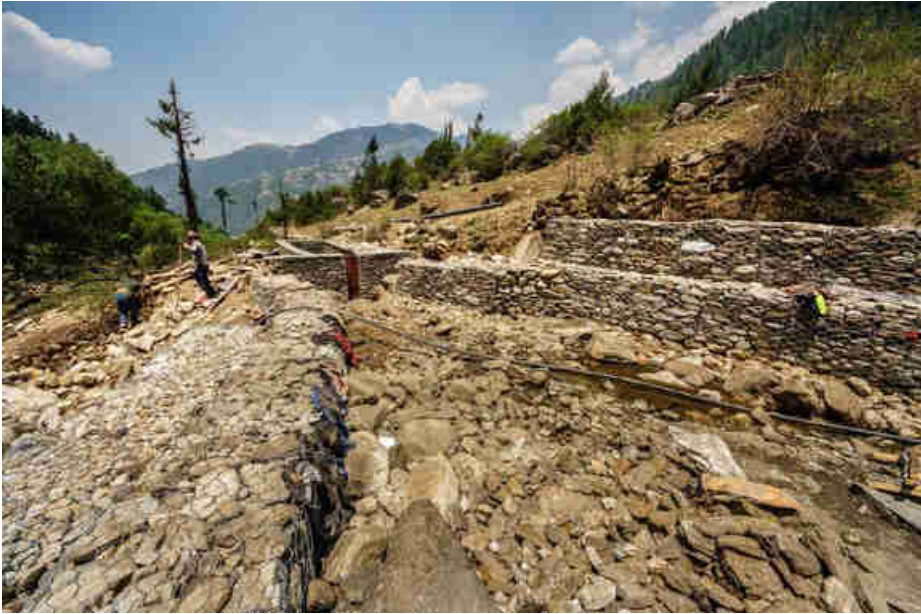
Pic. 91: Gabon wire boxes protection for the sluice gate and sedimentation tank
