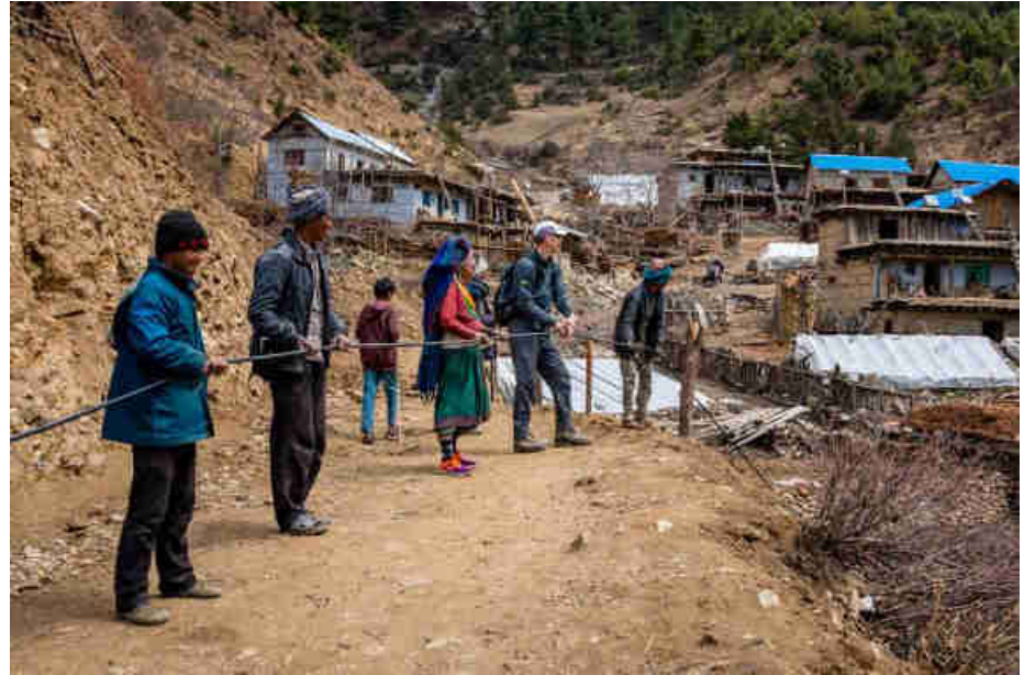
Pic. 28: Laying into the ground the cable from the turbine to the power house
