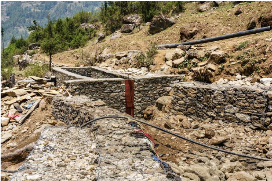
Pic. 93: Gabon wire boxes protection for the sluice gate and sedimentation tank
