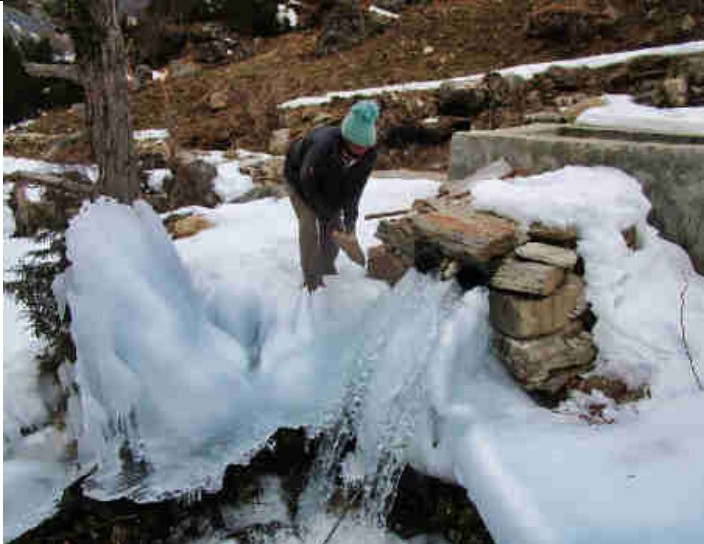
Pic 19: Water overflow HDPE pipes of the sedimentation tank are being check and made sure they are not blocked by the ice building up all around by the operator
