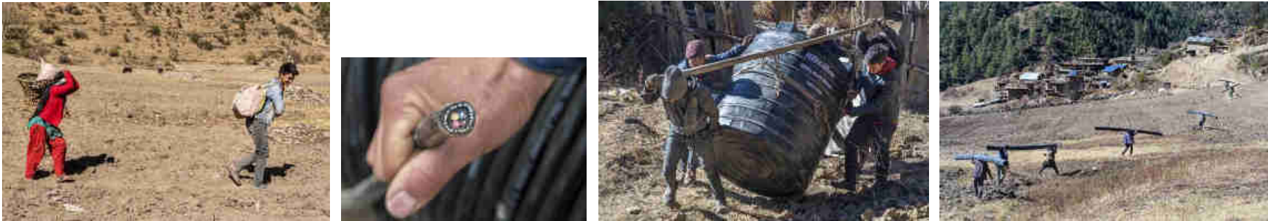
Pics. 33-36: From Mohari Village all the equipment and materials had to be carried by the Mohari people to the power plant site as there is no road or path beyond the village.
