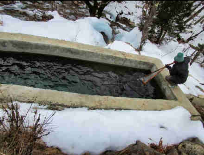
Pic 21: Periodical cleaning of the surface water from leaves and sticks in the sedimentation tank by the operator
