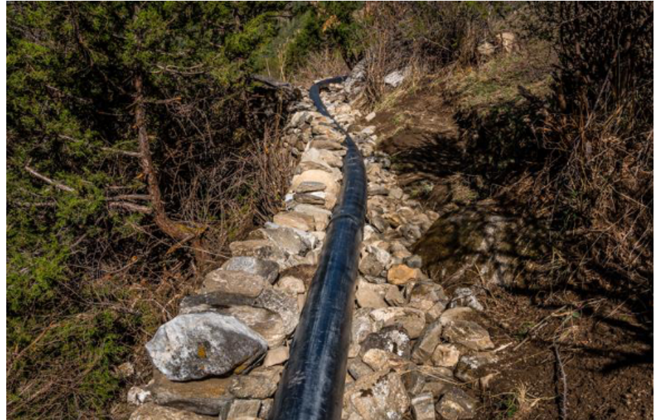
Pic. 56: The HDPE penstock is laid on soil and stone bed for protection
