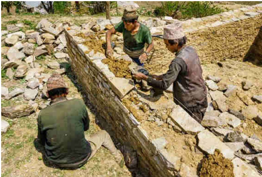
Pic. 109: Building the power house ground walls with stones and mud mortar
