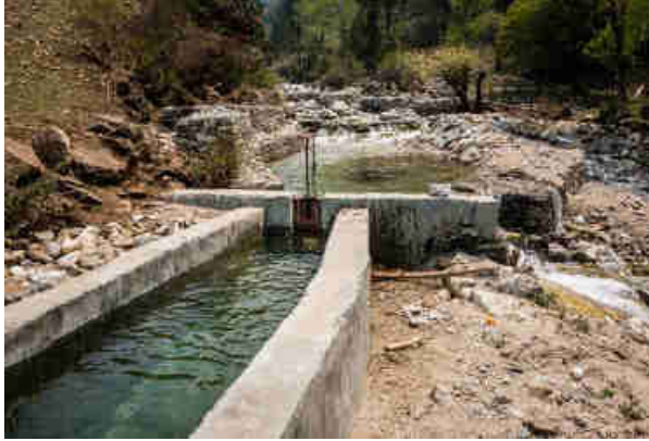
Fig 1: Two Levels of Sedimentation Tanks
