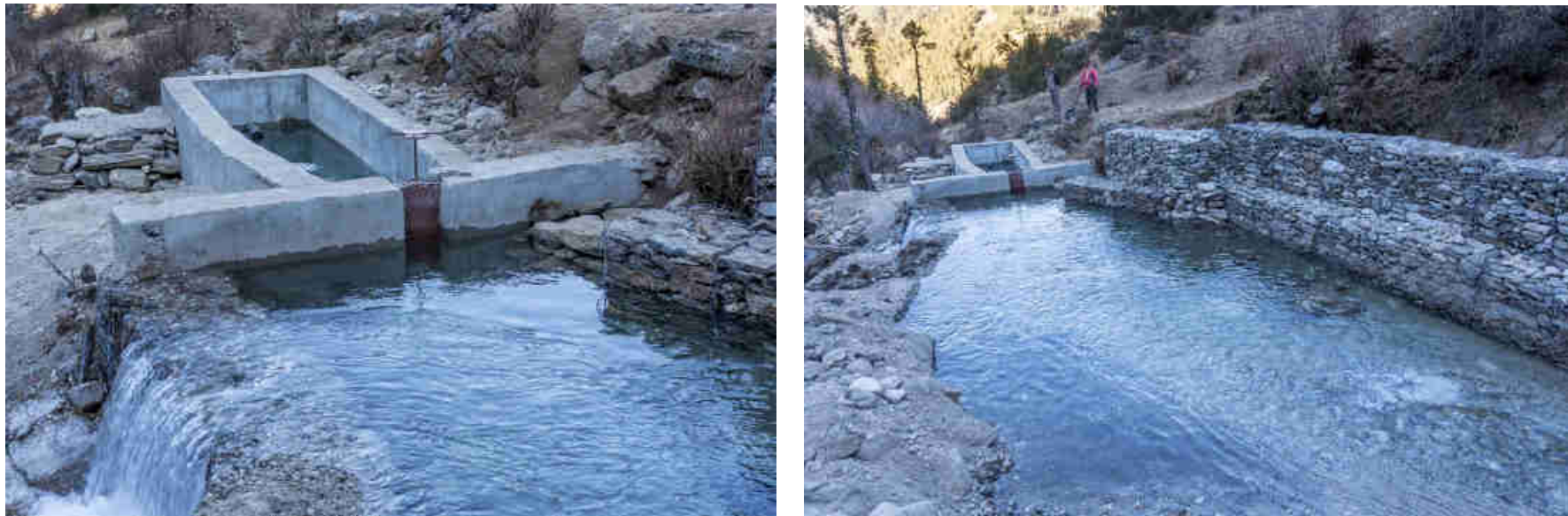
Pic. 13-14: After cleaning up the boulders and wooden logs the pond, intended to slow down the water flow for increased sedimentation of water, sand and silt is again working as intended. In that way the sedimentation tank and the pond in front of it provide very clean water to feed into the penstock to power the 6 Pelton turbines.
