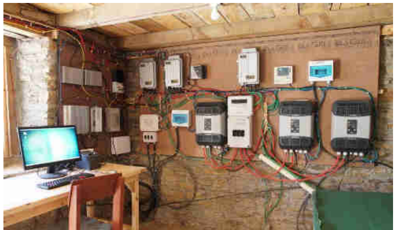
Pic. 16: Power house room where the 300 m long underground transmission line from the turbine house enters. Here is all the DC-AC power conversion equipment and battery bank. The PC serves for data monitoring/recording and issuing the monthly pre-paid codes for each user.
