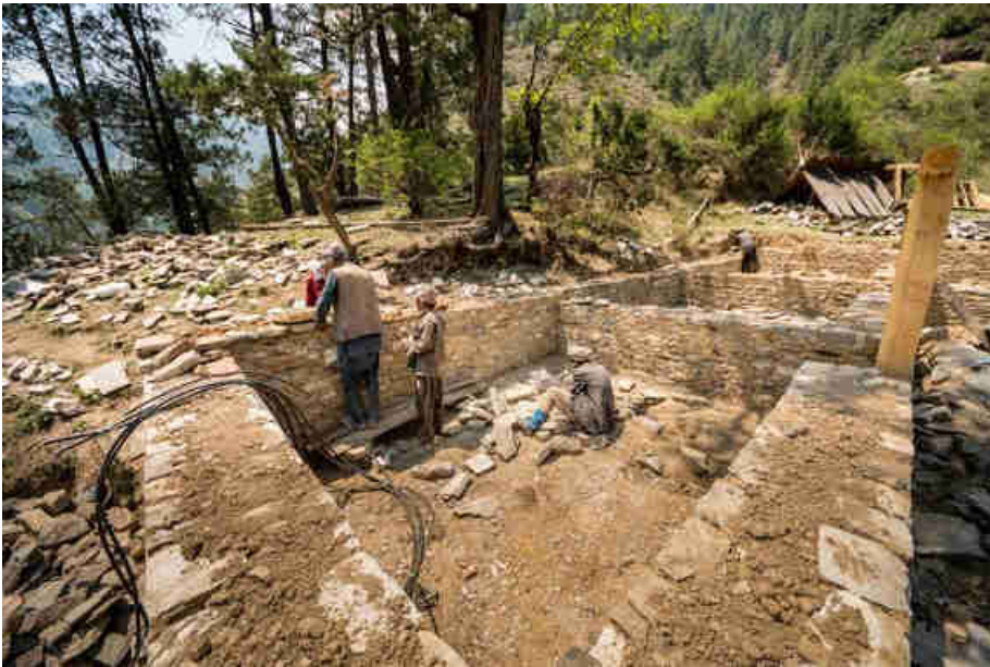
Pic. 113: Building the walls of the power room of the power house ground walls
