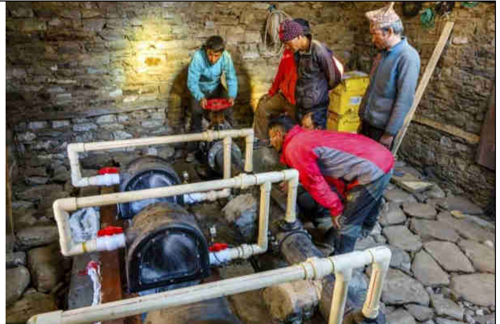
Pic. 27: Operator training: Correct start & stop of the power system is crucial
