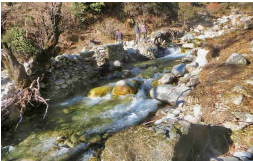
Pic. 1: Stone walls protect the created pond and sedimentation tank (left of stone walls) from boulders rolling down the river, especially during the rainy season.
