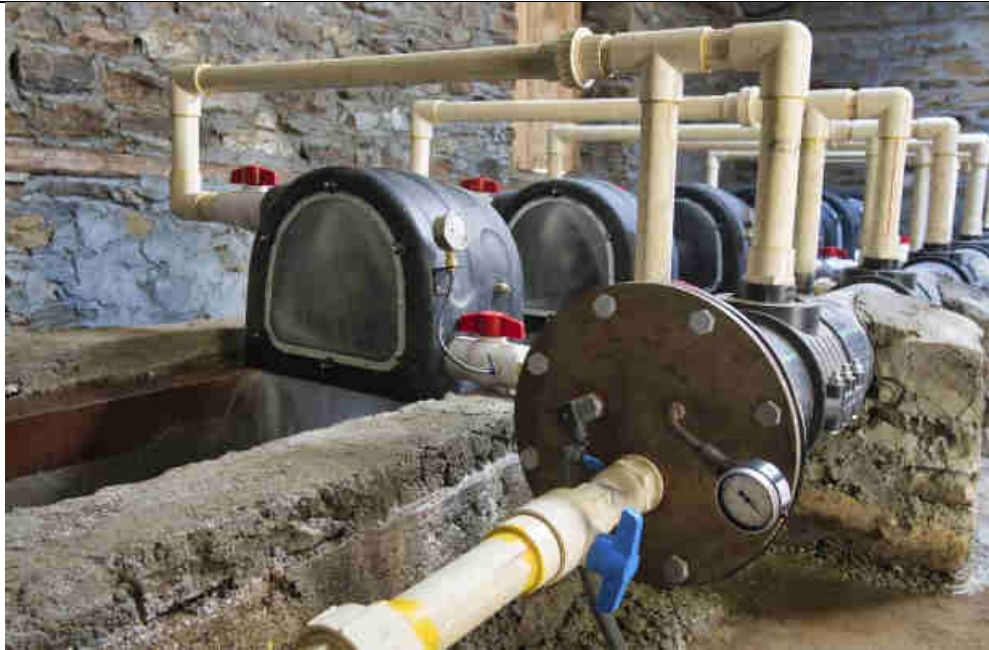
Pic 15: End cap of the 490 m HDPE penstock with a maximum Net Head of 47 m. Analog and digital pressure gauge are mounted to monitor the net head
