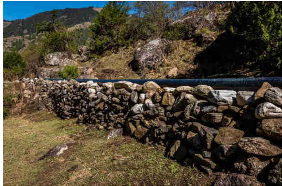
Pic. 54: HDPE penstock over a stone bridge for a gradual slope
