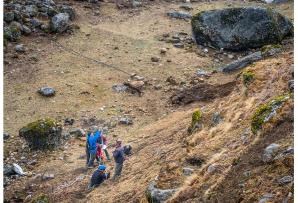
Pic 3: The last part of the penstock has a high drop of 20 meters
