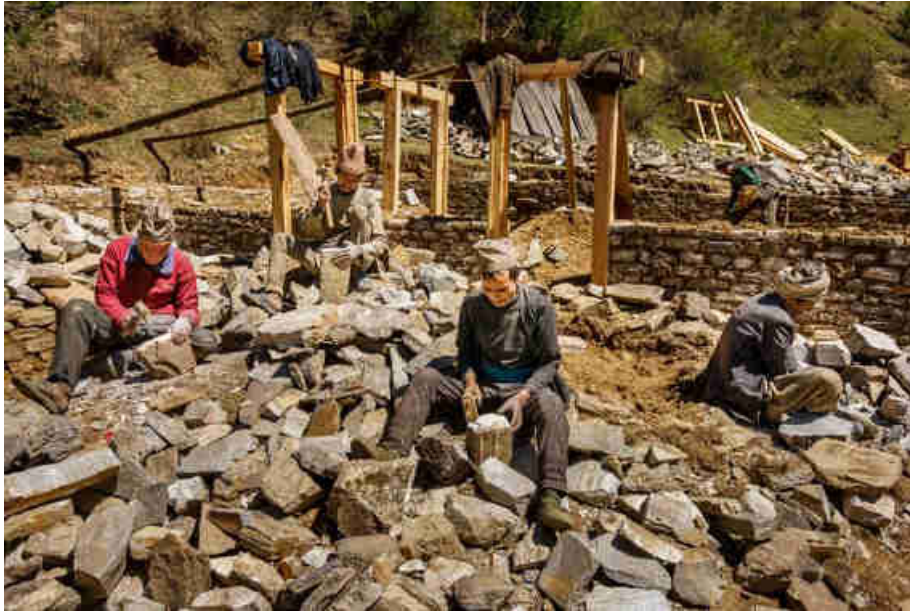
Pic. 107: Mansory work by the local men for the power house walls
