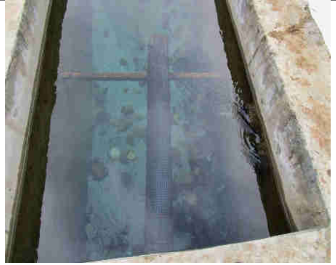
Pic 20: HDPE water filter pipe in the sedimentation tank which cleans the water running down the 460 meter long HDPE penstock to the Pelton turbines from any debris which could damage the turbine runners
