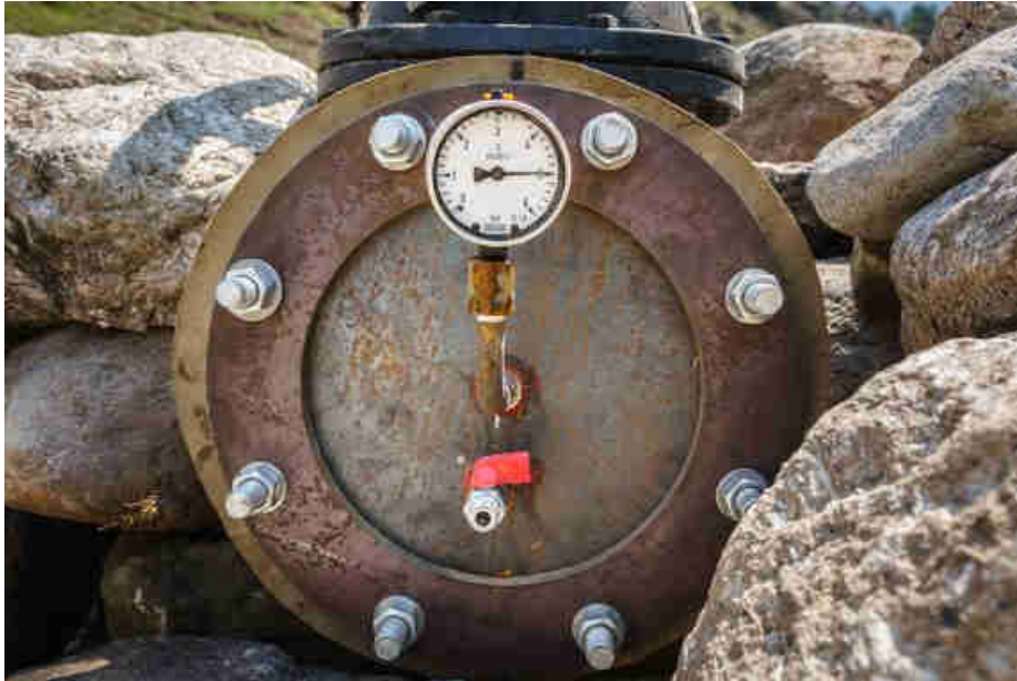
Pic. 67: Pressure at the entry of the turbine house is exactly 5 bar or 50m head
