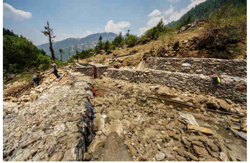
Pic. 15: Gabion wire boxes protection for the sluice gate and sedimentation tank
