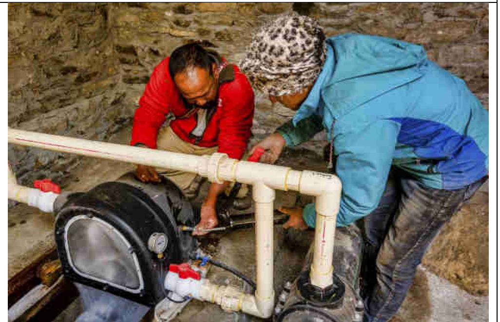
Pic 10: Monthly greasing of each turbine while it is continue to generate electricity
