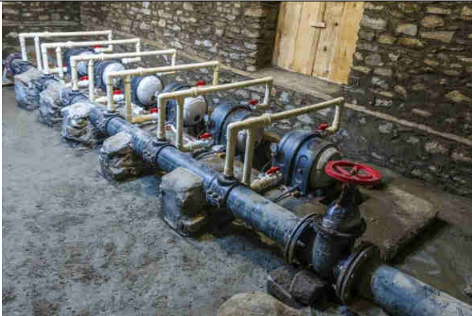
Pic. 30: Modular Pico-Hydro Power with 6 PowerSout Pelton Turbines installed
