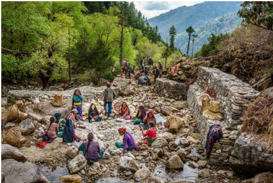
Pic. 81: The women crushing stones with a hammer for gravel for the cement
