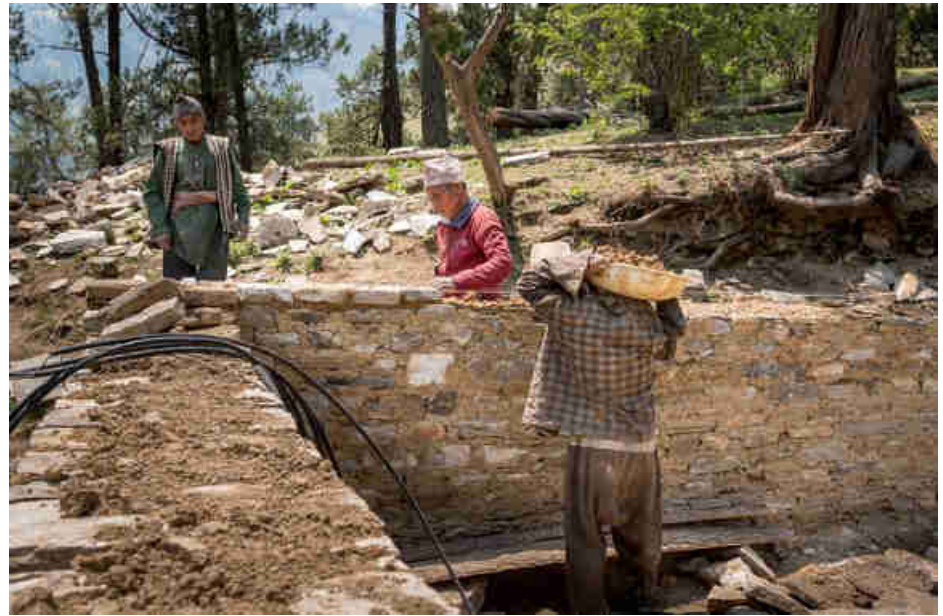
Pic. 122: Building the ground floor walls of the power room in the power house
