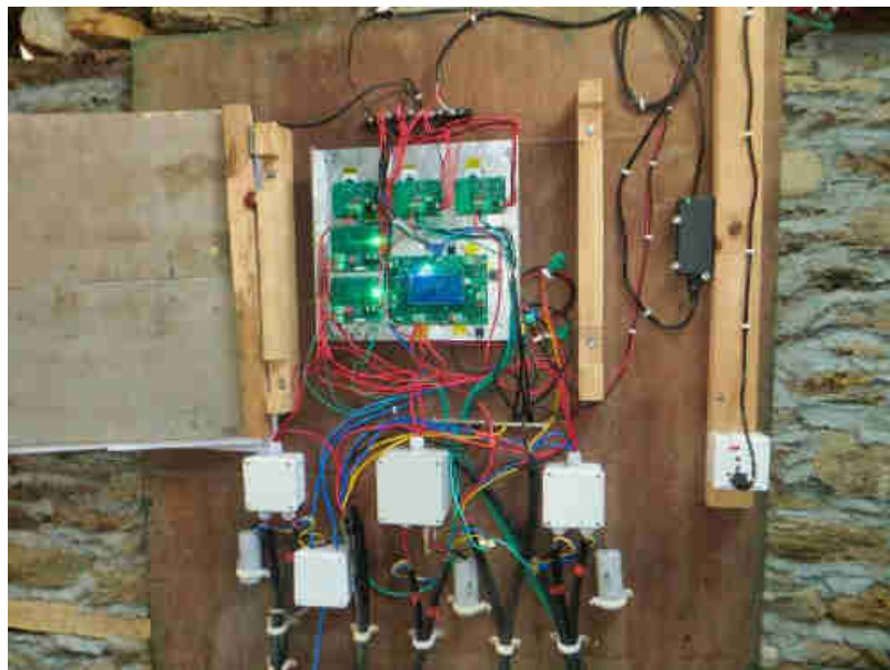
Pic. 13: Mother board and DC power cable connection in the turbine house, to get the 300 VDC power transmitted via the 300 m long, 60cm underground buried, armored cable transmission line, to the village.
