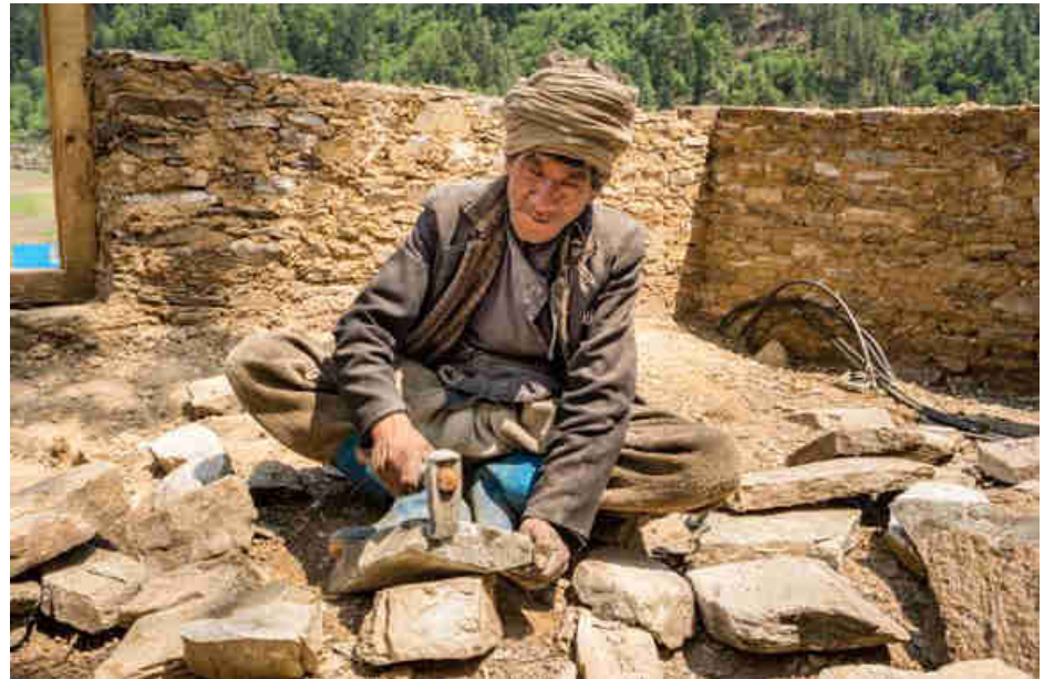
Pic. 114: Masonry work for the walls of the power room of the power house
