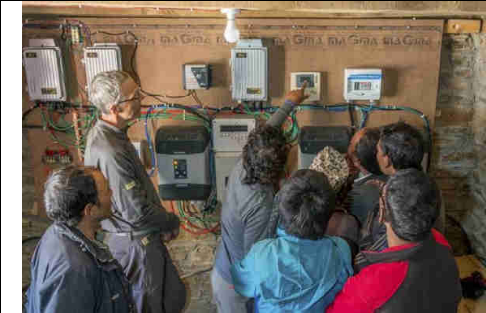
Pic. 26: Operator training for correct O&M of the power system in the power room
