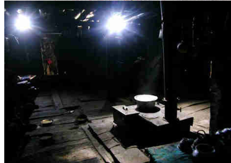
Fig. 8: Installation of a 20 watt Solar PV home system on the mud roof of one of the Mohari families homes, with two of the three 1 watt white LED lamps in their main room.
