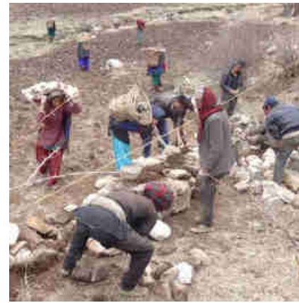
Fig. 14: Building Elevated Penstock
