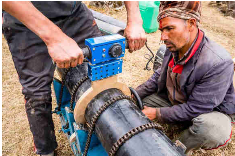
Pic. 38: Joining the 200mm HDPE penstock pipe with the heating plate (220° C)
