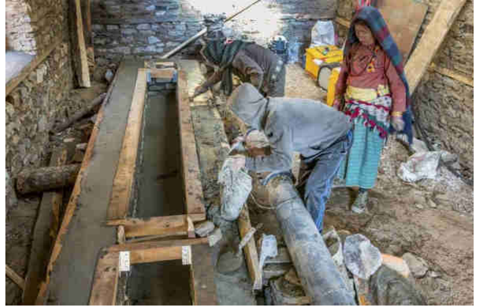
Pic.19: Building the water canal for the 6 Pelton Turbines inside the turbine house
