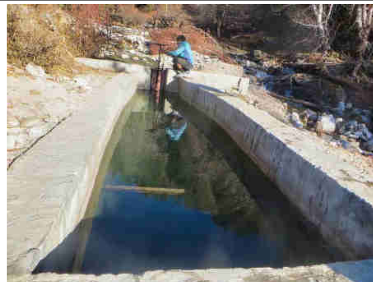
Pic. 4: Hiralal, one of the two trained pico-hydro power plant operators from Mohari, adjusts the gate valve to let water flow slowly into the sedimentation tank from the pond, so that all the sand and impurities can fall out, before the water is led into the penstock.
