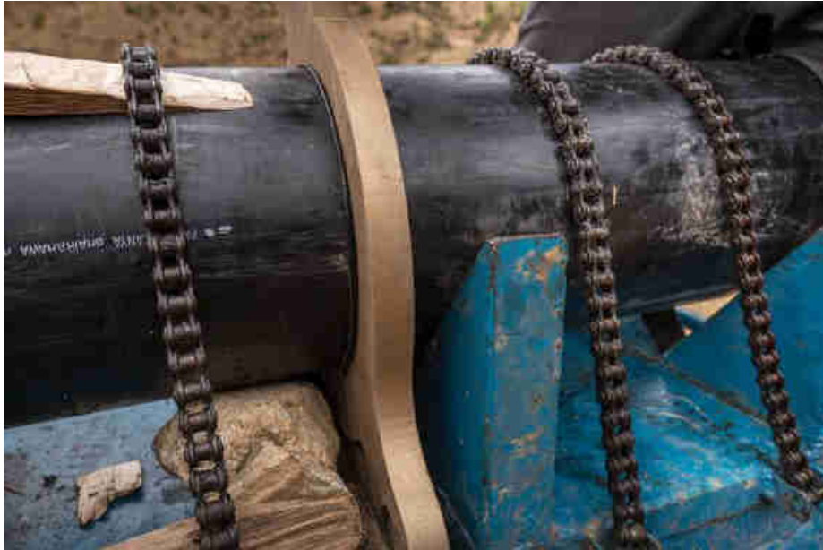
Pic. 39: The HDPE pipes are held in place with chains to assure straightness
