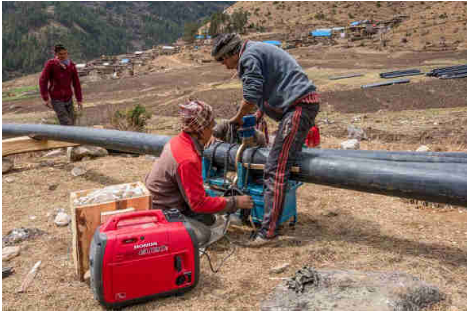
Pic. 35: Joining the 200mm HDPE penstock pipe with the heating plate (220° C)
