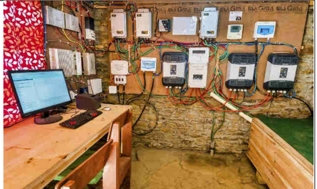
Pic 64: The modular pico-hydro power plant’s power room in the P/C house with the village power distribution, DC/AC conversion and battery bank, able to provide e.g. for AC motor start starting time (<5sec) up to 15 kW power from a 6.6 kW hydro power plant. That enables income generation activities such as a carpentry workshop
