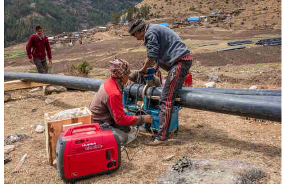
Pic. 7: Joining the 200mm HDPE penstock pipe with the heating plate (220° C)
