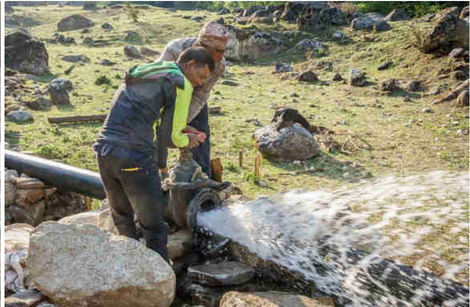
Pic. 70: Release of the water in the 455 m long penstock HDPE pipe
