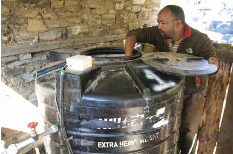
Pic. 38: Checking the hot water tank of the village warm/hot shower center
