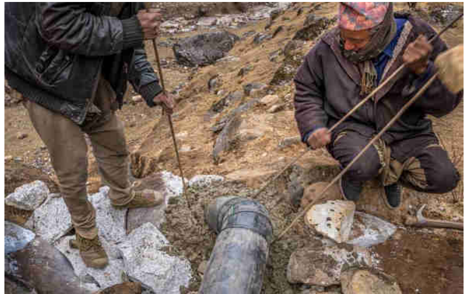
Pic. 50: The 45° elbow of the steep drop is anchored and secured with cement
