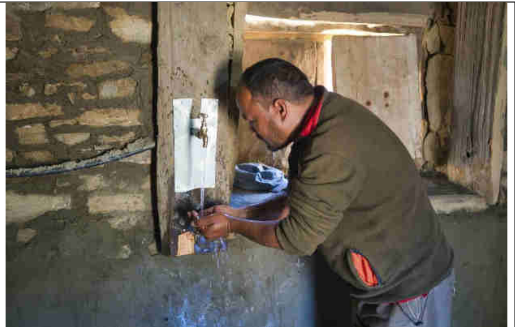
Pic 44: Hot water tap in the village shower room for operator to cleaning the shower
