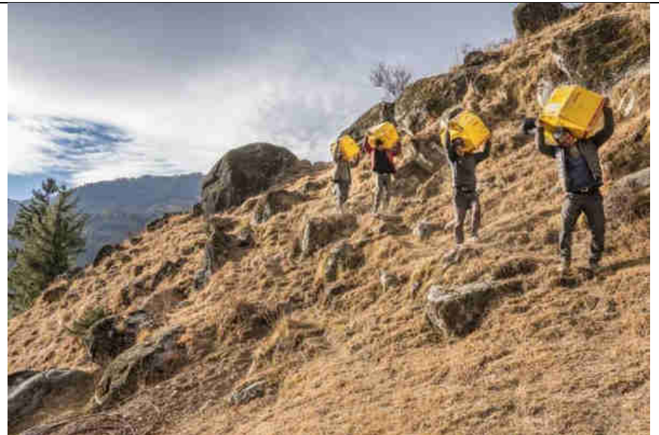
Pic. 21: With no roads the 6 Pelton Turbines and all equipment had to be carried
