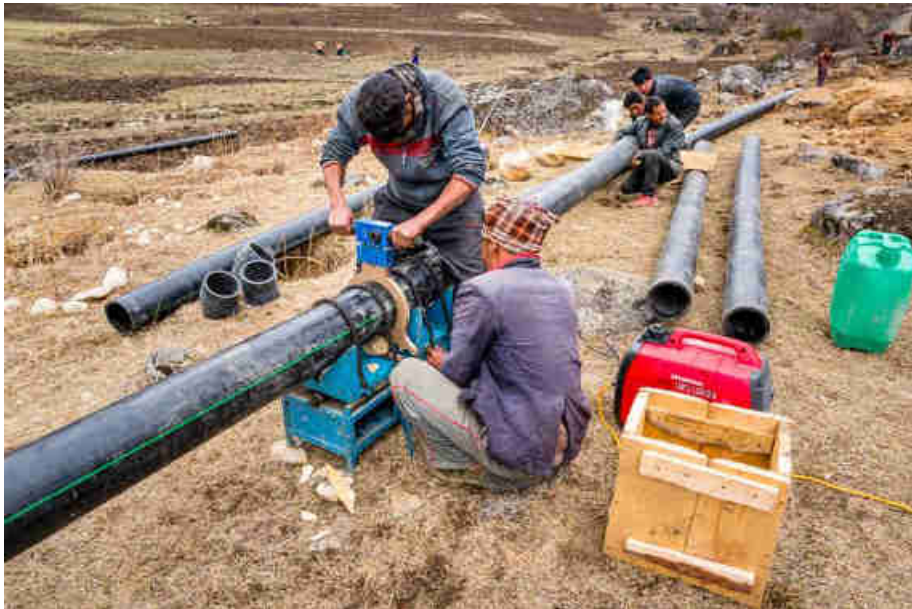
Pic. 41: RIDS staff trained local people to weld the HDPE pipes together
