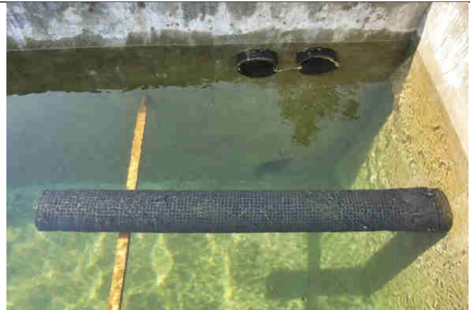
Pic. 25: Intake water filter and HDPE overflow pipes in sedimentation tank
