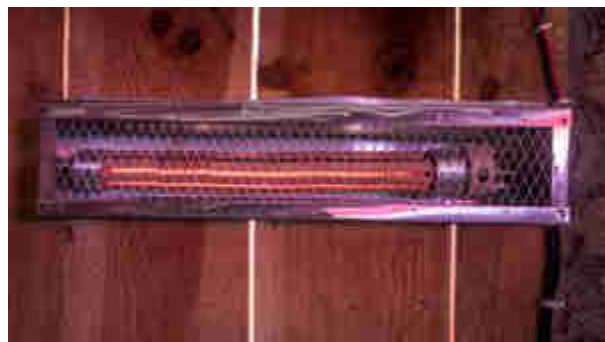
Fig. 12: Air Heater Resistor in the Community Center
