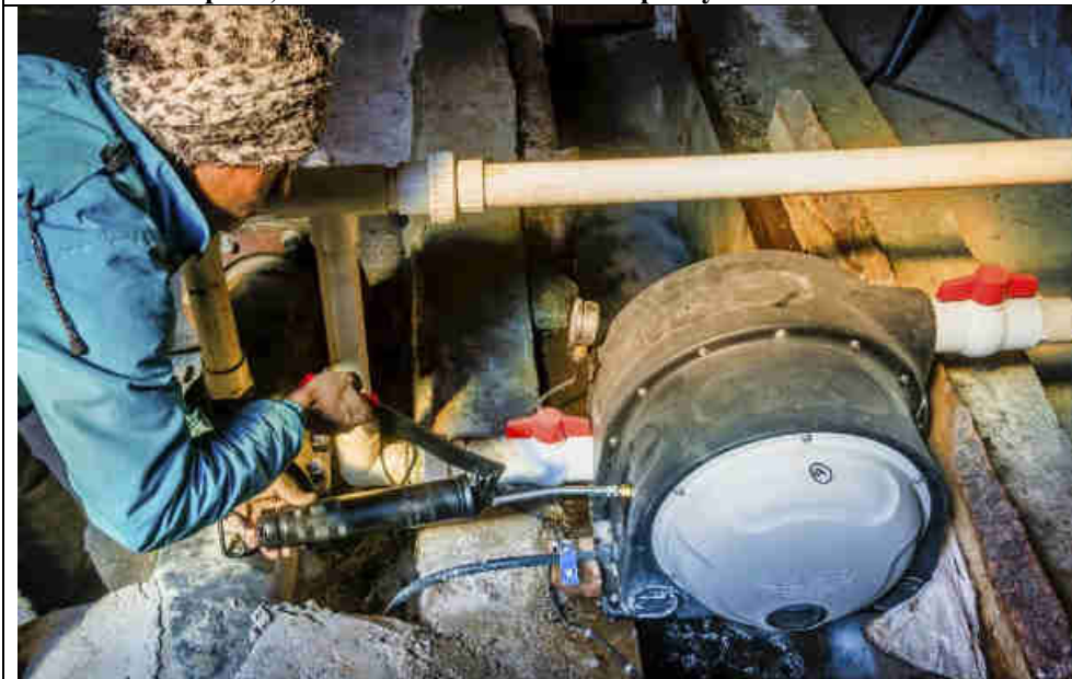
Pic 9: Monthly each turbine is greased as part of the periodical maintenance while the turbine is running producing its expected power output
