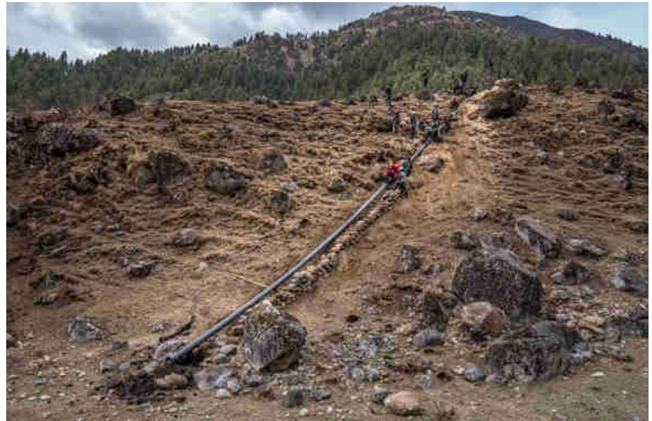
Pic. 66: The last, steep sloped HDPE penstock pipe before the turbine house
