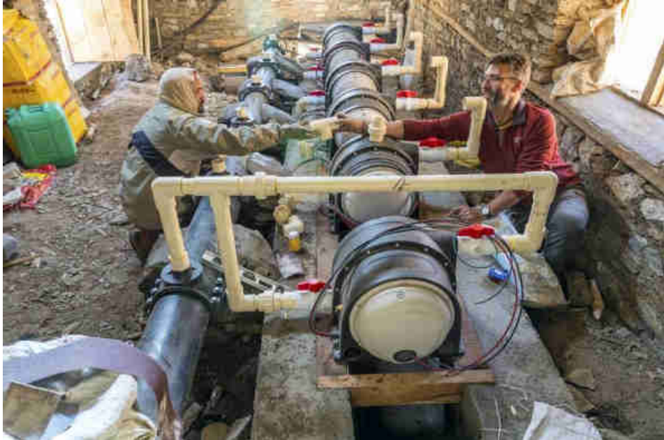
Pic. 22: 2" PVC piping installation to connect all the 6 turbines to the HDPE penstock
