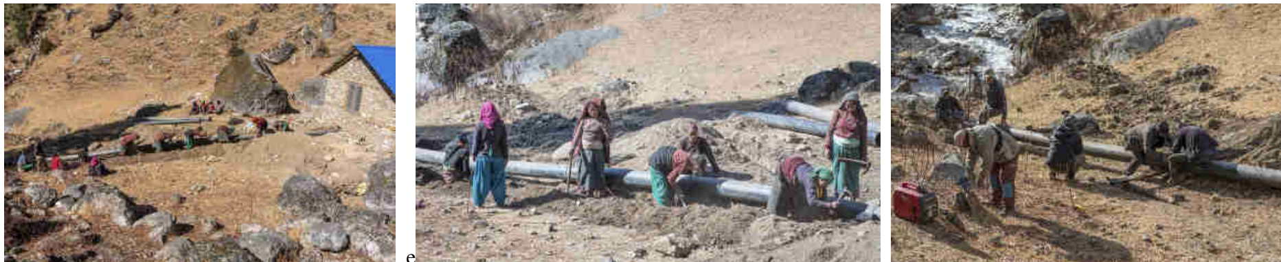
Pics. 79-81: Under the direct supervision of the RIDS staff the Mohari village families are digging and buidling the 30 m long, underground buried, Modular Pico-Hydro power plant water outflow HDPE pipe (225m diameter PN2.5), to lead the water used to generate the power back into the river.
