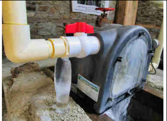
Pic 2: Pelton Turbine 1 of 6 forming icicles under the nozzle ball valve. The river water temperature is just under 1° Celsius
