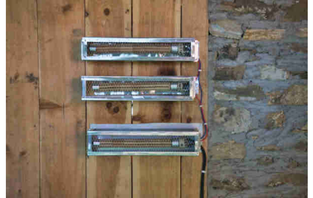
Pic 62: Room heating (one of the various “smart dump loads”) to increase the indoor room temperature during the cold 10 months in the P/C house for improved comfort
