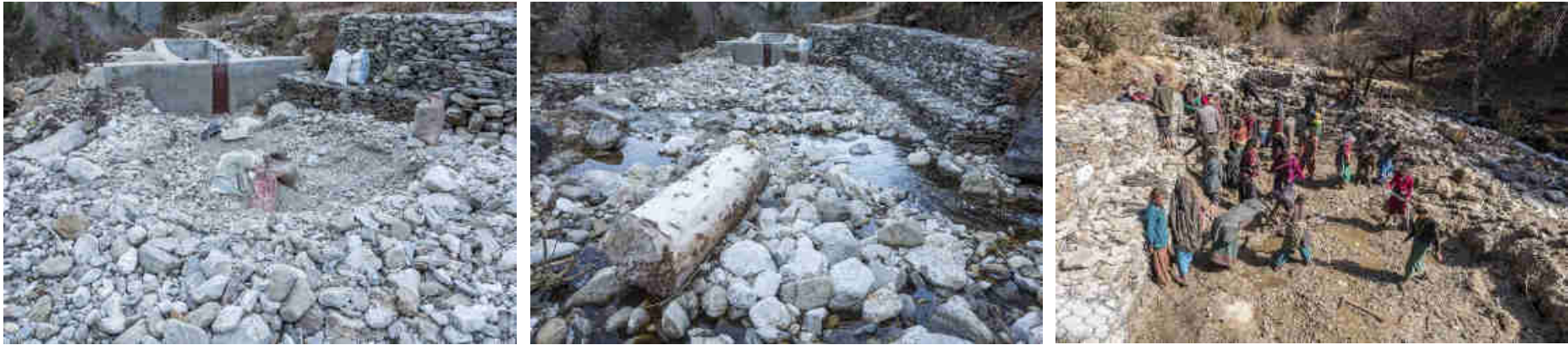
Pic. 10-12: After the heavy and long monsoon season from June - October (10 years height!) the built water pond was covered with boulders and tree logs. However the sedimentation intake was fully protected. In 2019 six more protective Gabon Wire cages will be built to protect the sedimentaion tank and pond even more.
