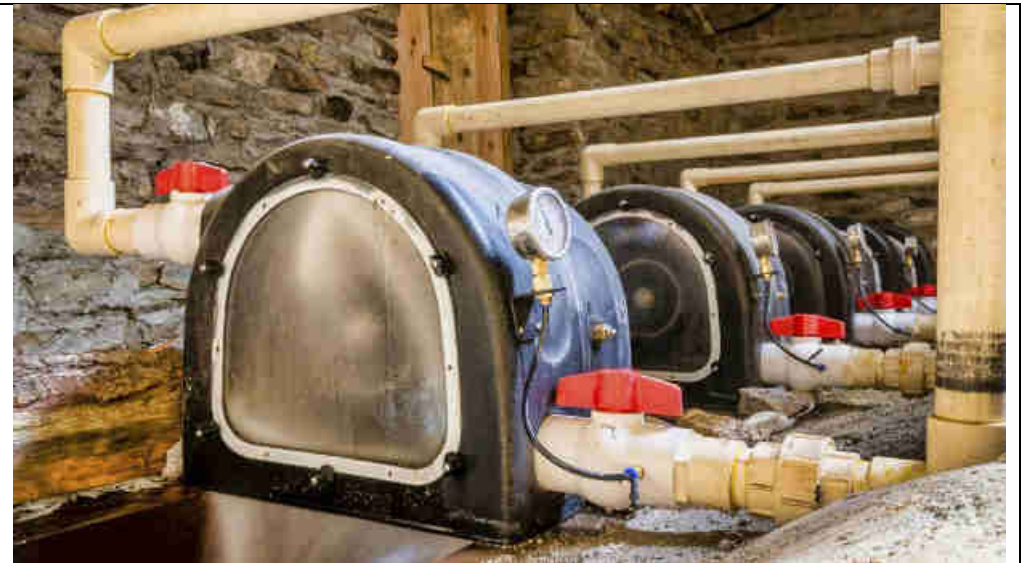
Pic 8: Every individual turbine can be shut down for inspection, maintenance or repair by simply closing its two ball valves (red handles) to cut the water flow to the two jets of the Pelton turbine. The other turbines continue to produce electricity.
