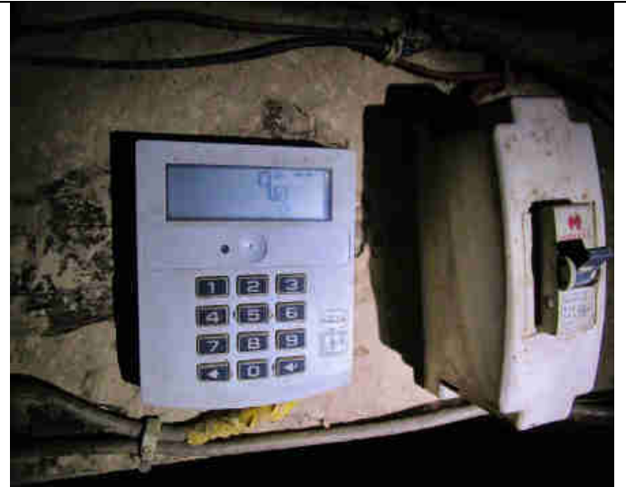
Pic 8: Input panel (left) for the code for the monthly pre-paid electricity units plus the security fuse (right) inside the home for safety
