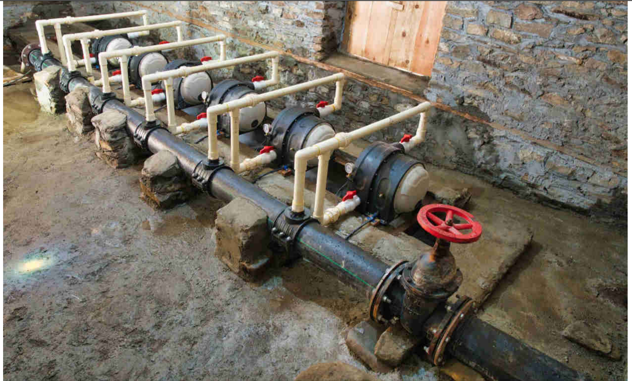
Pic 6: The 6 PowerSpout Pelton turbines in the modular pico-hydro power plant turbine house. A 490 m long, 200 mm HDPE penstock pipe, half a meter underground buried, brings the clean water from the sedimentation tank down to the turbines. The DN200 16 bar Gate Valve is adjusted to the needed head (max. 47m) and water flow (max. 20L/sec) to regulate power generation. The modular pico-hydro power plant can generate from 300 W (one turbine at 30%) to 6.6 kW (6 turbines 100%), based on the village's power demand. Thus initially one turbine is sufficient, with additional turbines added, "growing dynamically" with the village's increasing power demand over the years.
