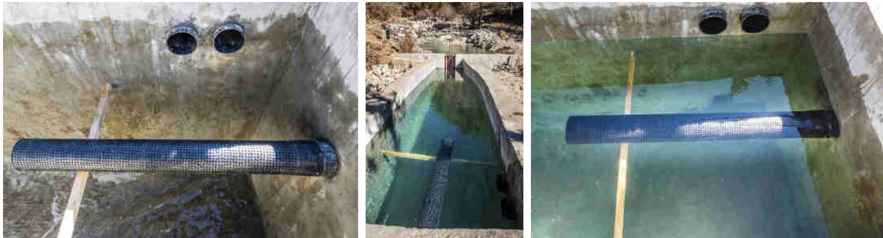
Pics. 88-90: Installed new HDPE 200 mm diameter Intake water filter with 1060 x 8mm holes plus the two 180 mm diameter HDPE overflow pipes, with the sedimentation tank, shown empty and filled. The washout is at the bottom right if the sedimentation tank. It enables to flash out the collected sand and silt constantly out of the sedimentation tank, improving the protection of the Pelton turbines at the end of the 460 m long penstock HDPE pipe.
