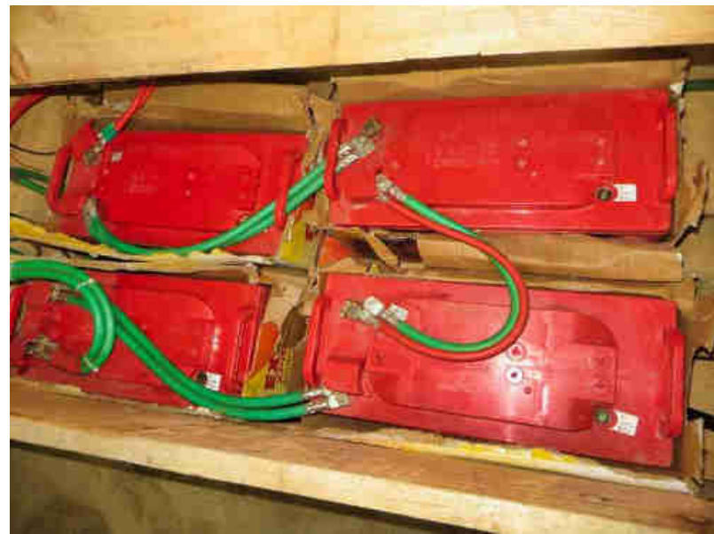
Pic. 14: 48 VDC battery bank in the village's power house. The battery bank allows the DC/AC inverters to provide 3-phase AC power with up to 30 sec. 12 times the power plant's rated output power e.g., to start a motor.
