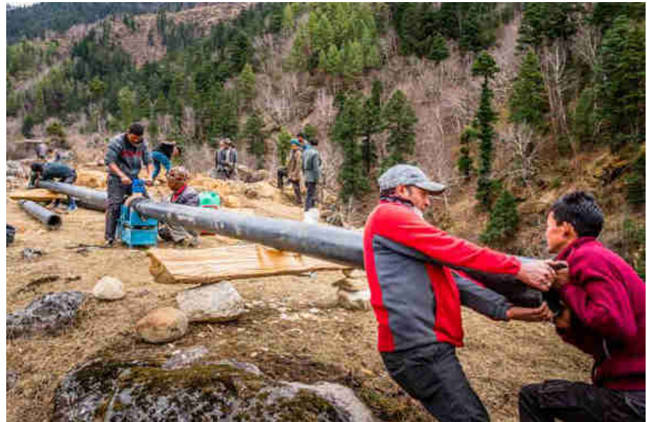
Pic. 42: All local people are part in welding the HDPE pipes for the penstock
