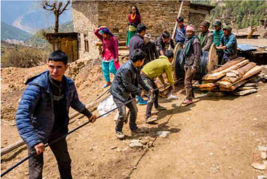
Pic. 27: Unrolling the underground cable from the turbine to the power house
