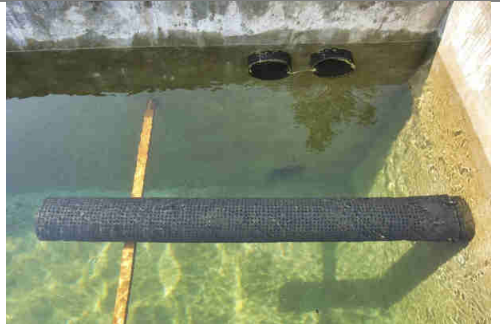
Pic 24: Cleaned HDPE intake filter at the sedimentation tank and overflow pipes
