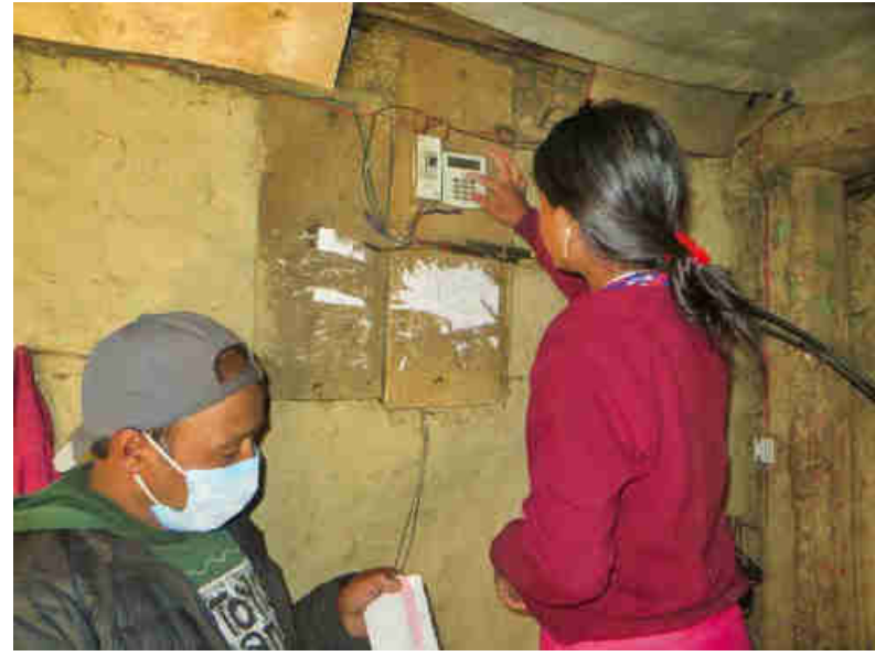
Pic. 22: RIDS-Nepal staff, Mansingh is helping a woman to recharge her meter box with the 20-digit number on the token issued by the pre-payment system.
