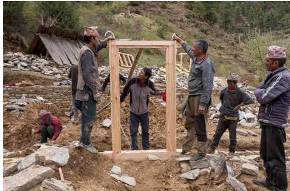
Pic. 102: Installing the first ground level wooden door of the power house
