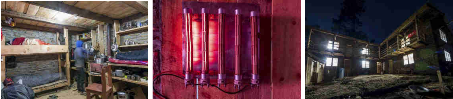
Pics. 125-127: Power/community house kitchen (left), “smart dump load” resistor 48 VDC room heater (middle) and the 2 floor, power/Community house with light in each room.
