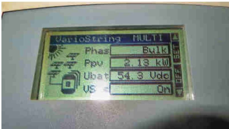
Pic. 15: Two of the six Pelton turbines, at 40m gross head and ~7.5 L/sec water flow generate 2.13 kW AC in the village. That results in a system efficiency from water to AC electricity of around 72%. The battery bank is close to max. voltage at 54.3 VDC.
