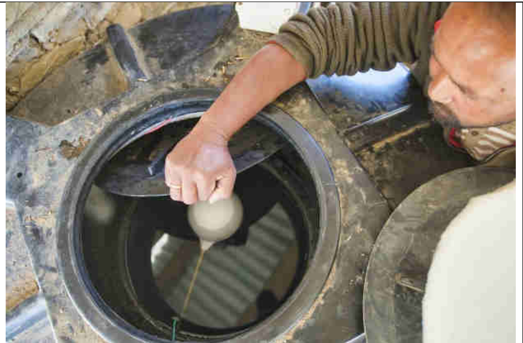
Pic 40: Checking the intake ball valve of the hot water tank warm/hot shower center
