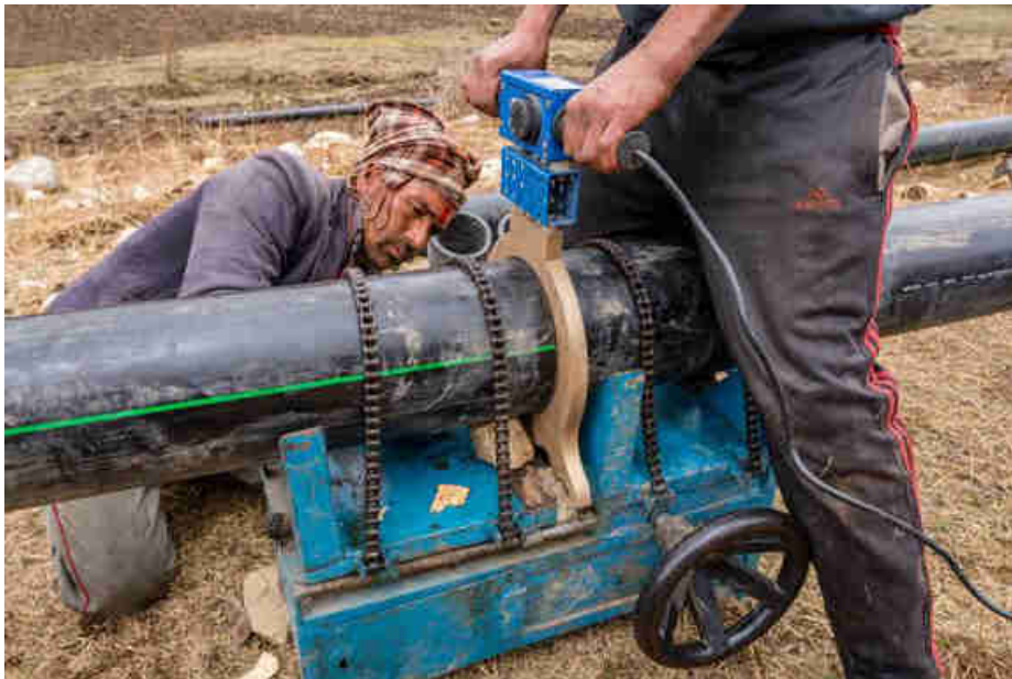
Pic. 37: Joining the 200mm HDPE penstock pipe with the heating plate (220° C)
