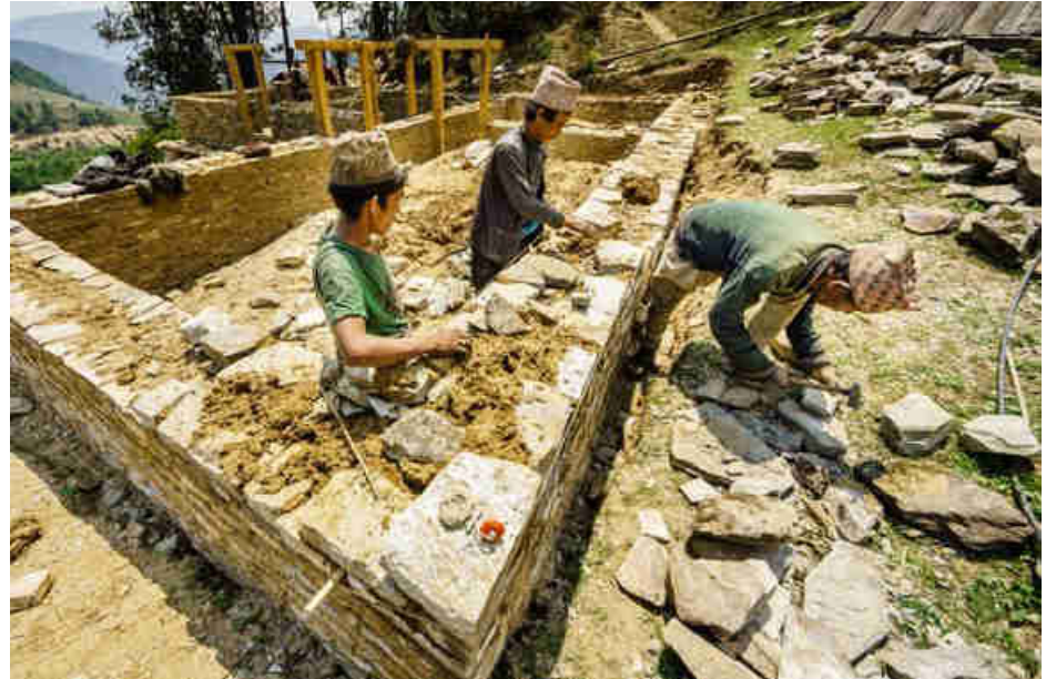
Pic. 112: Building the power house ground walls with stones and mud mortar
