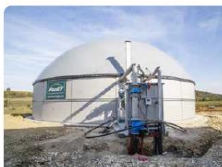
Day 10: Installation and commissioning of the membrane roof with gas storage. Gas and minor supply lines connected.
