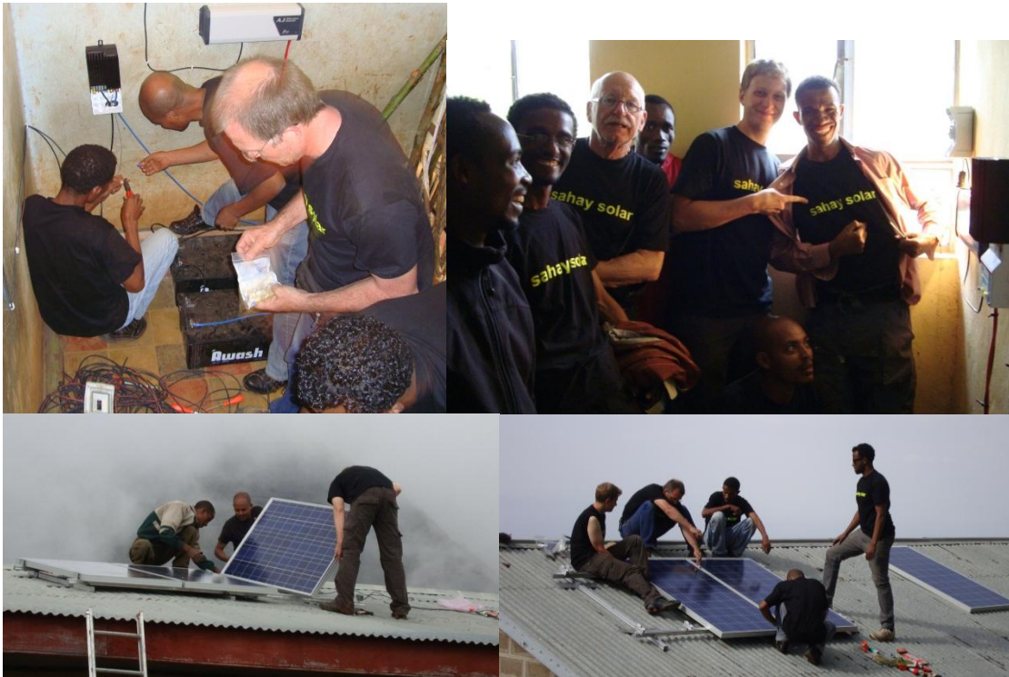
Installation of PV systems at rural village schools in the Arbaminch region
