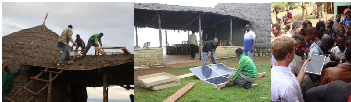
Installation of a PV system at Dorze Lodge by locally trained professionals from AMU SCC | Sales of Pico SHS in Danbile
