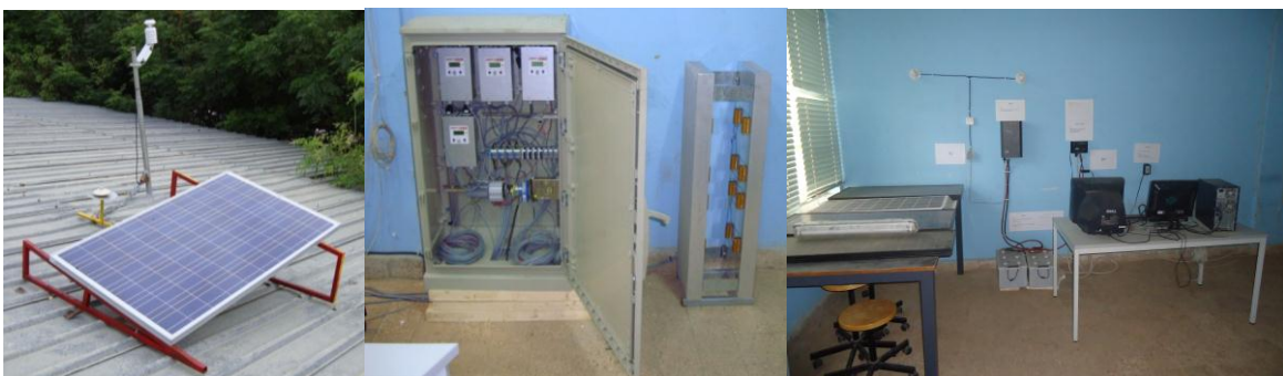
PV testing system, MPPT data acquisition box and PV laboratory at AMU SCC
