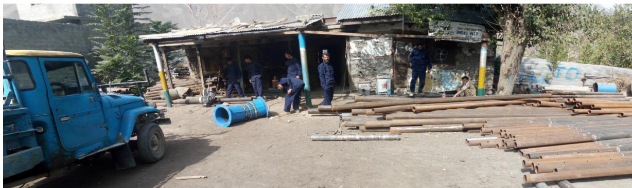
Figure 6 MRSC Welding plant
