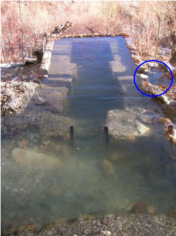
Picture 6.6 Flooded forebay tank
