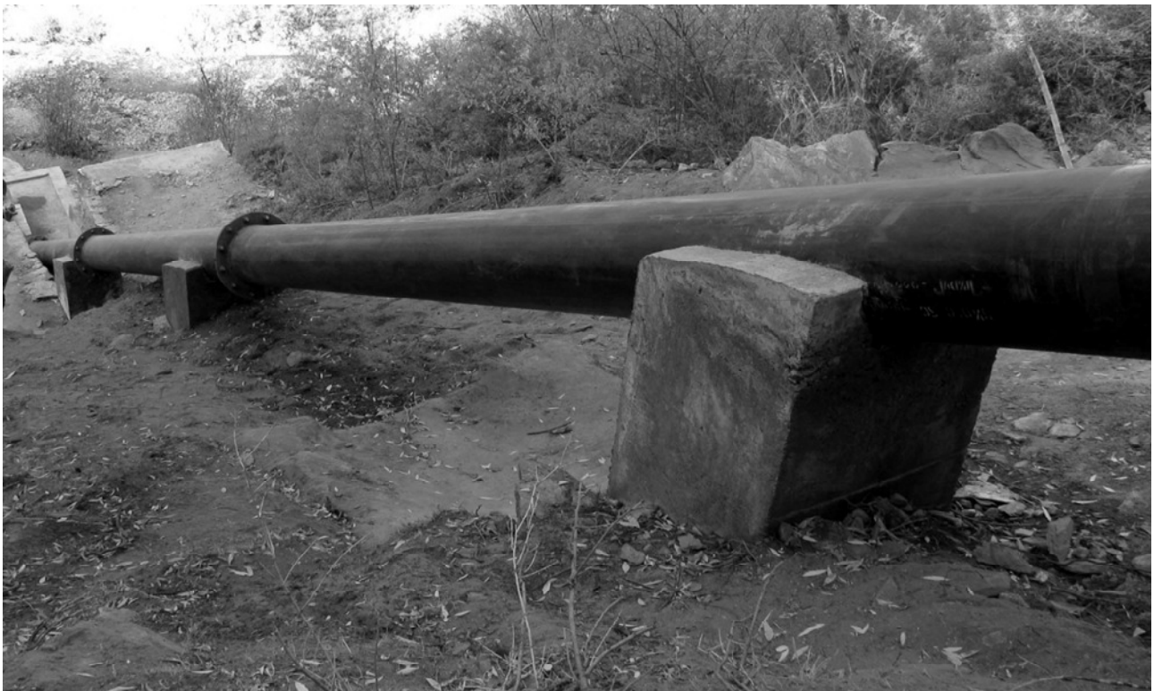
Figure 7.9 Mild steel penstock on sliding blocks
