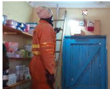
Figure 8. First customers receive electricity service.
