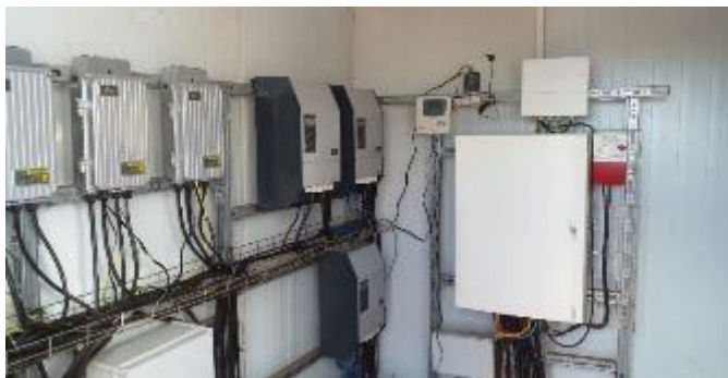
Figure 9. Technical house interior (inverters, charge controllers and meter).
