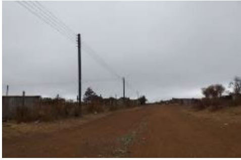
Figure 4. One of the 3 phases line of the grid network
