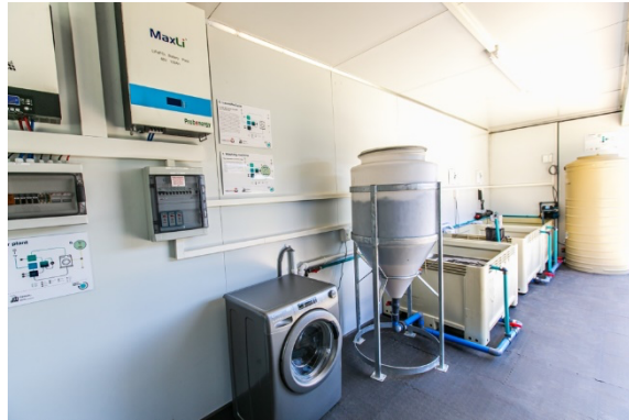
Figure 8: Interior of the LaundReCycle pilot plant including washing machine and installations for the water treatment
