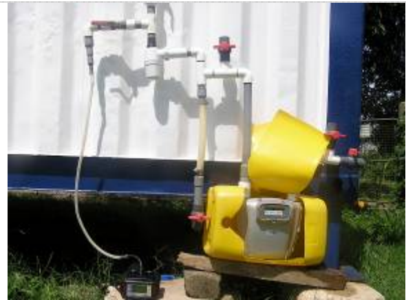
Picture 10. Installation for gas measurements
